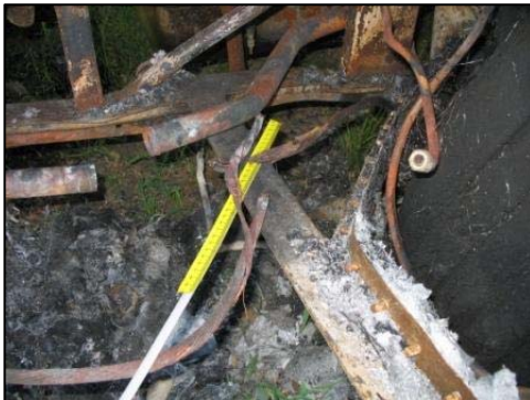
Figure 16. Arced and separated battery cable.
