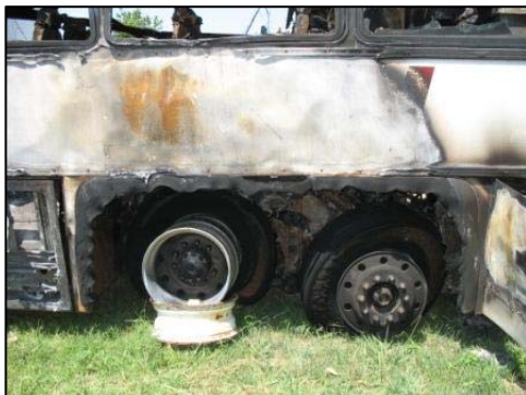
Figure 8. Fire damage to the left drive and tag axle tires and wheels.
