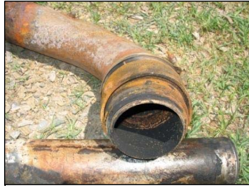
Figure 13. Exhaust pipe removed from turbocharger.
