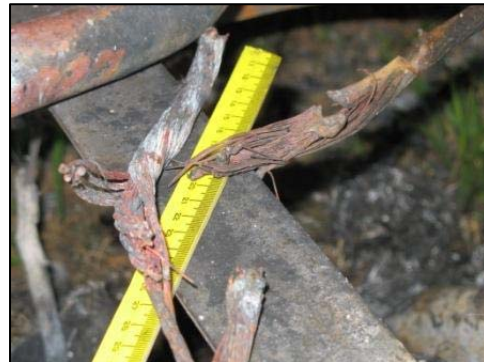
Figure 17. Close-up view of the arced cable.
