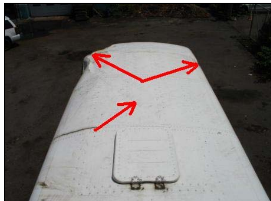
Figure 12: Roof damage from towing activities.
