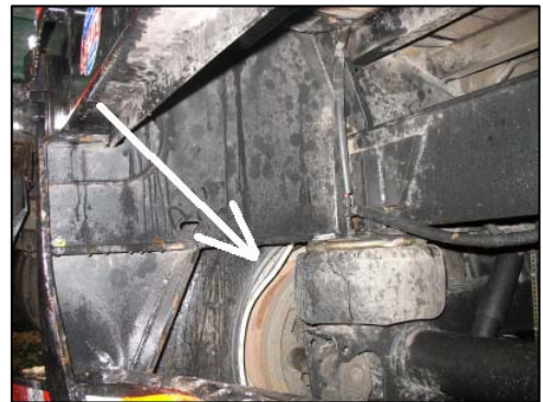
Figure 9: View of the deformed inboard left rear wheel rim.
