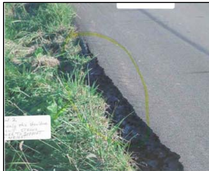
Figure 3 - Fractured road edge.
