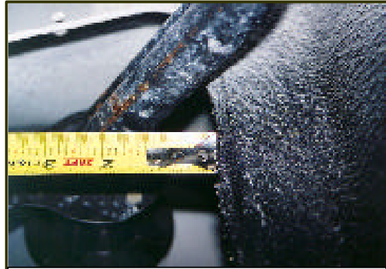
Figure 17. Close-up view of the proximity of the filler tube to the inner fender edge.
