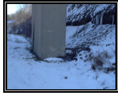
Figure 4. Point of impact - concrete bridge support
