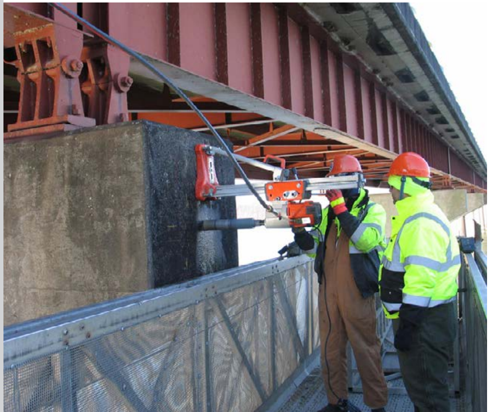
An inspection of the John Coffee Memorial Bridge, part of the Natchez Trace Parkway over the Tennessee River.
