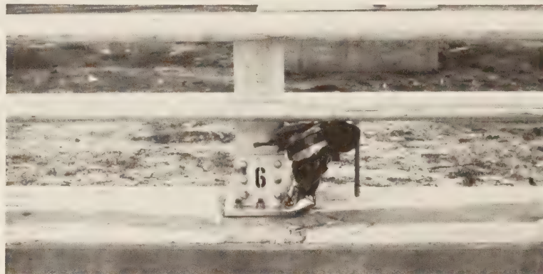
Figure 11.—New Hampshire bridge rail after crash tests.
