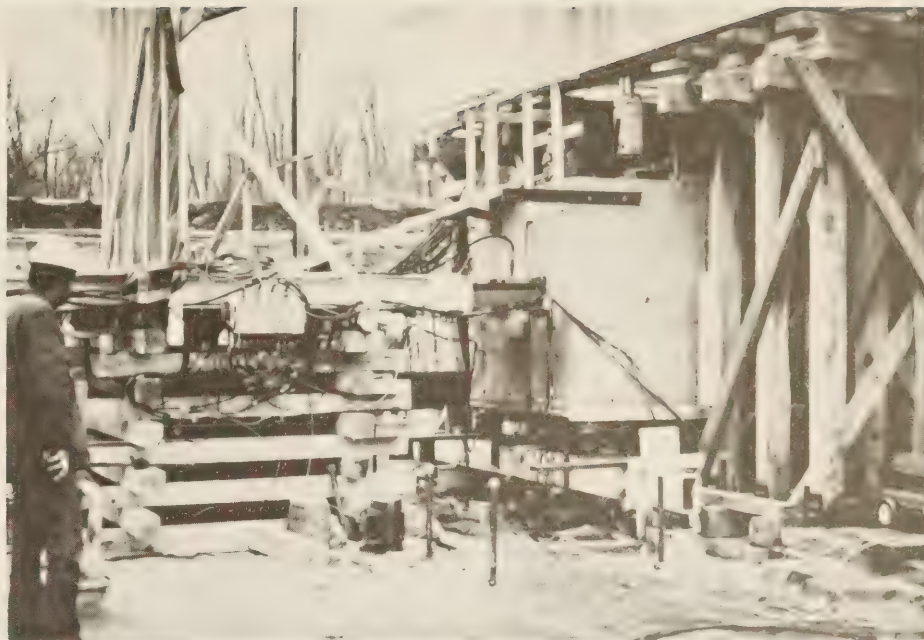
Figure 4. —Pile load test on group of eight timber piles at Locks and Dam No. 26 near Alton, Illinois.
