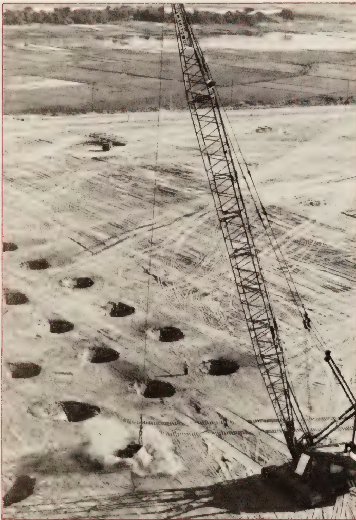
Figure 6. — (a) Second pass of heavy tamping weight being dropped by 100 ton (91 Mg) crane to dynamically compact loose foundation soils.
