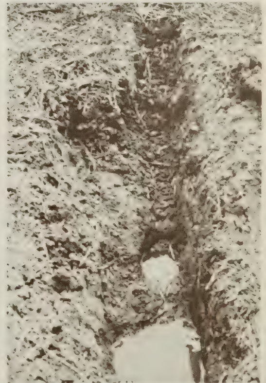
Figure 3.—Lack of positive outlets for drainage layers causes underdrain deficiencies.
