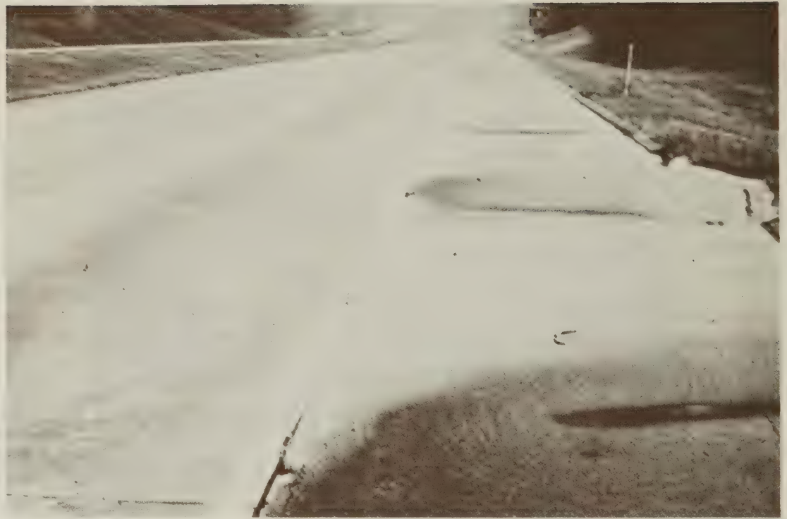
Figure 1.—Water seepage from joints and cracks downgrade from inflow source.
