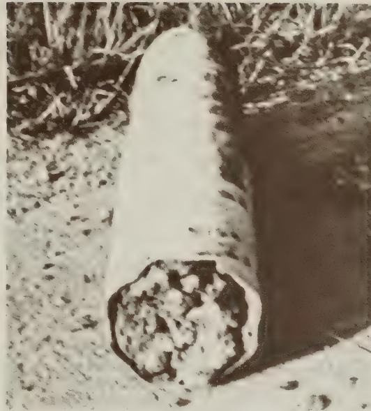
Figure 2.—Underdrain deficiency—clogged pipe.
