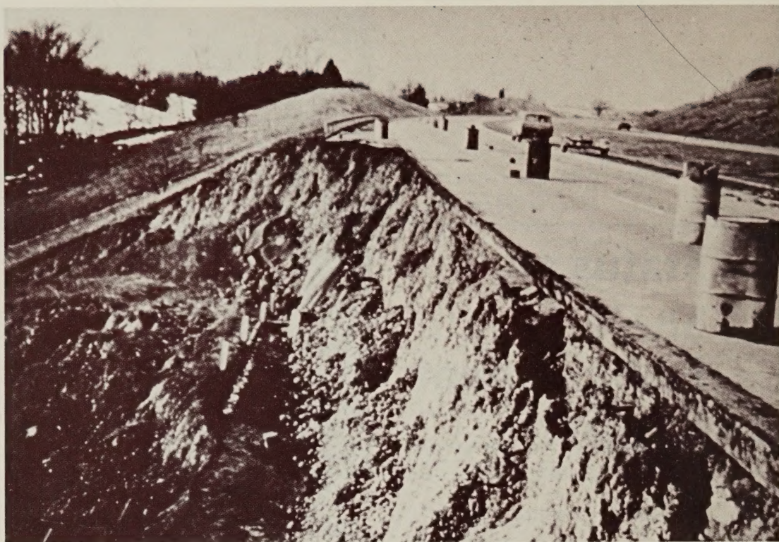
Figure 1.—Western portion of embankment failure on Interstate 74. —courtesy of the Indiana State Highway Commission
