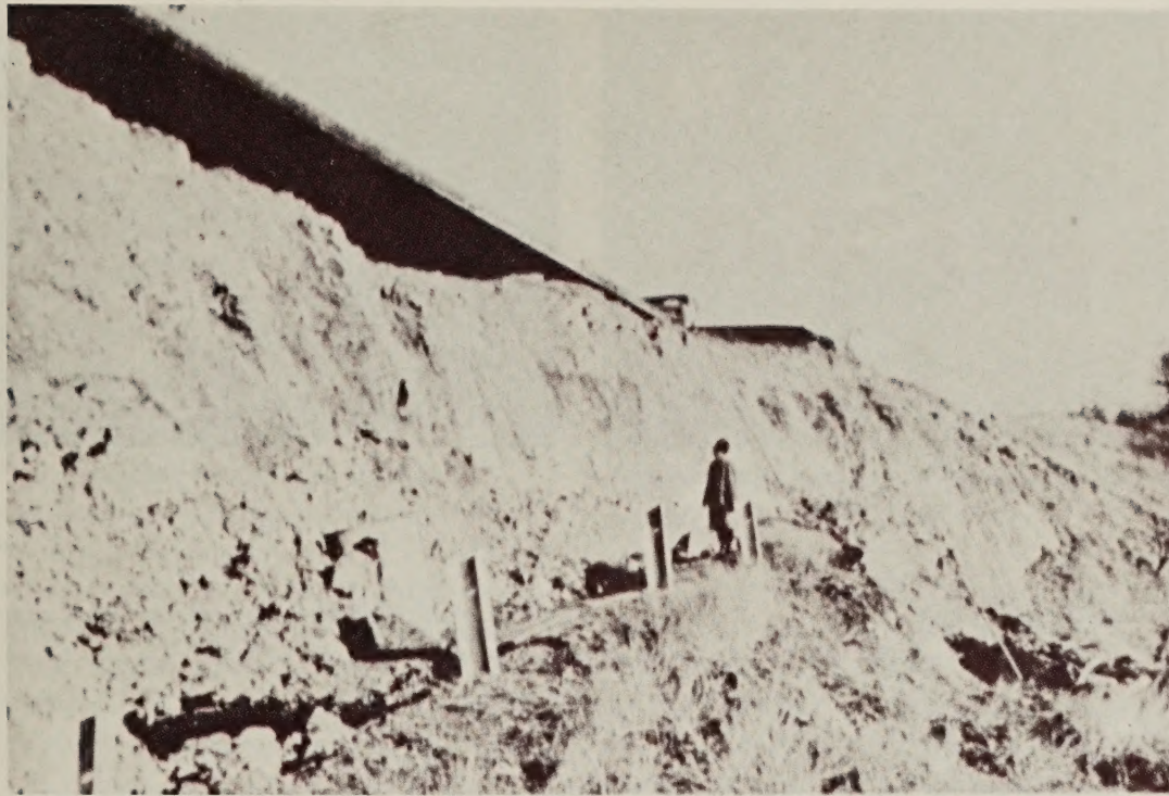
Figure 2.—Eastern portion of embankment failure on Interstate 74. —courtesy of the Indiana State Highway Commission
