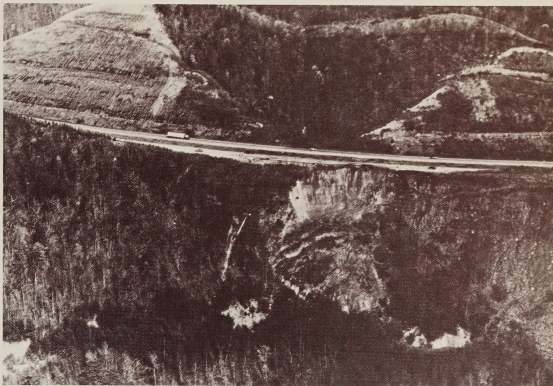
Shale embankment failure on Interstate 75 in Tennessee.
