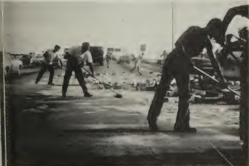
Figure 2.—Removal of debris on the roadway can cause traffic congestion and delay.
