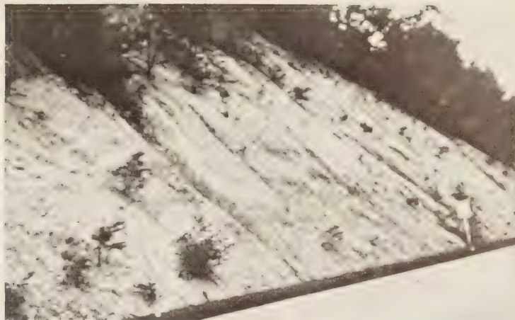
Figure 1.—Eroded cut slope.
