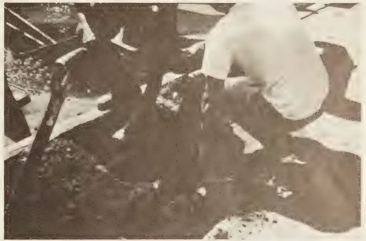
Figure 20.—Installation of bend from splice box in the direction of the manhole.
