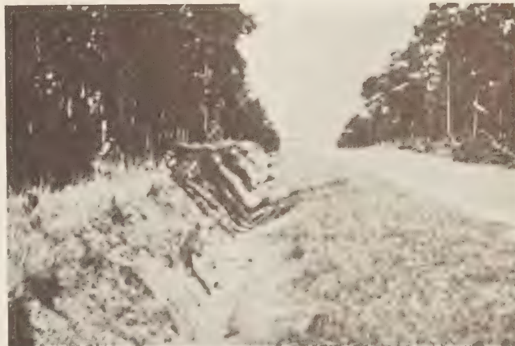
Figure 7.—Badly eroded ditch.
