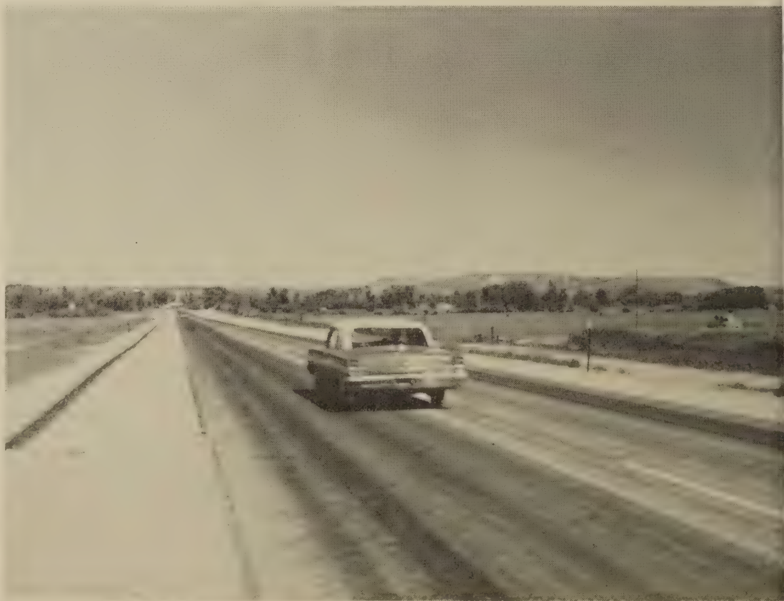
Figure 2.—Unsatisfactory (excessively rich) seal coat.
