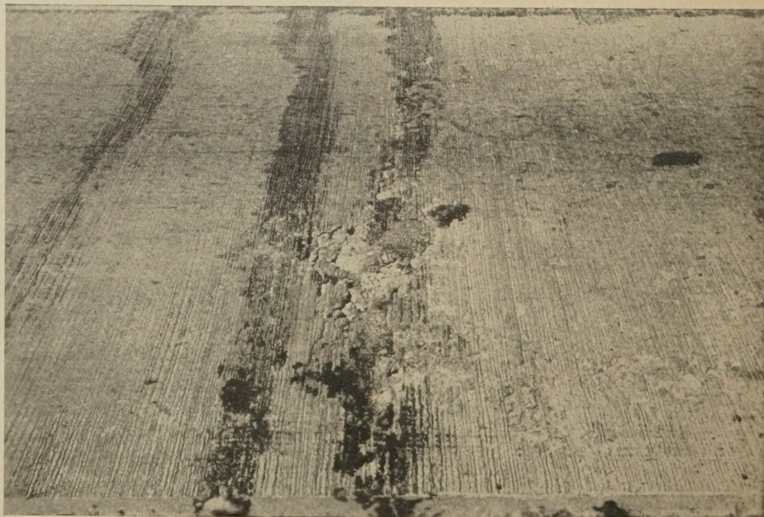
Figure 8.—Extreme case of spalling at a crack in a section reinforced with heavy steel bars. Even minor spalling at such cracks is unusual.
