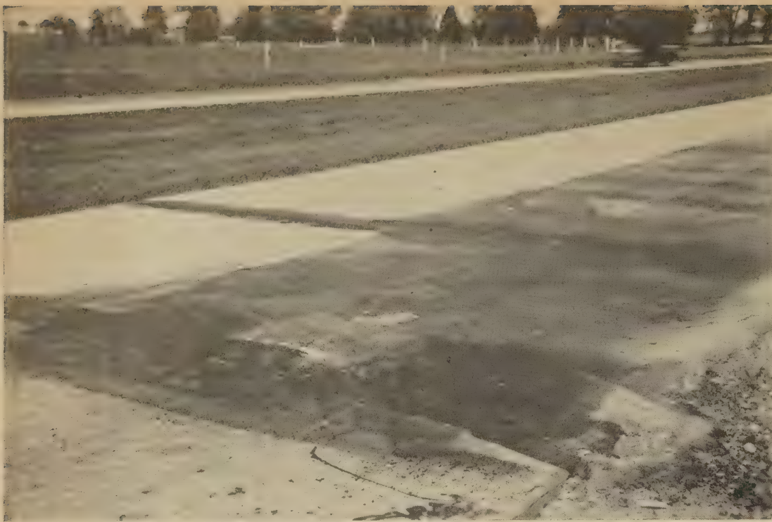
Figure 11. —Condition after 15½ years of a double bridge-type expansion joint, typical of the majority. Loosening of the steel cover plate, pumping, and faulting developed at an early age at most of these joints in the heavily traveled lane.
