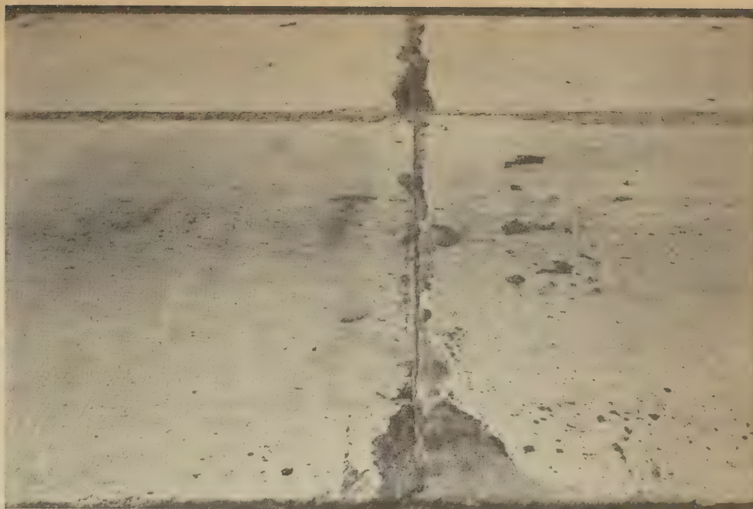
Figure 12.—Condition after 15½ years of a construction joint in sections reinforced with wire fabric. Tie bars were used to hold adjoining slabs together.
