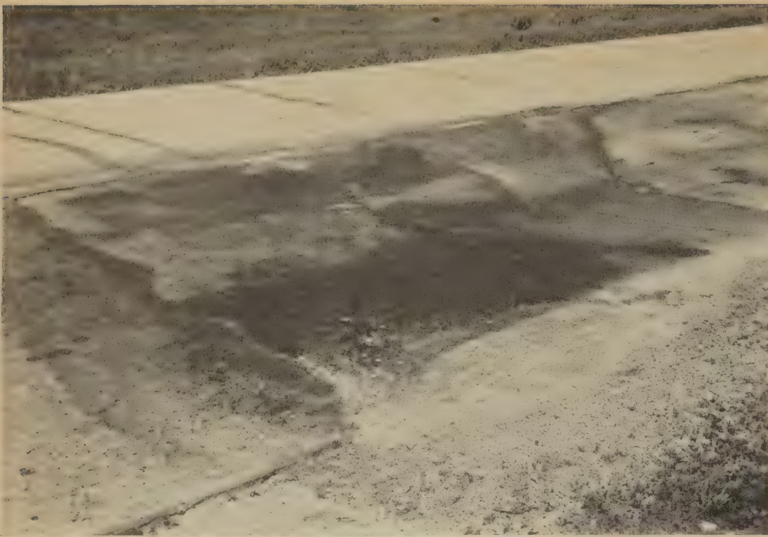
Figure 14. —Condition after 15½ years: Slab failure in heavily traveled lane near center of 830-foot section reinforced with 1-inch rail-steel bars. Faulting at longitudinal joint and edge pumping preceded structural breakdown.
