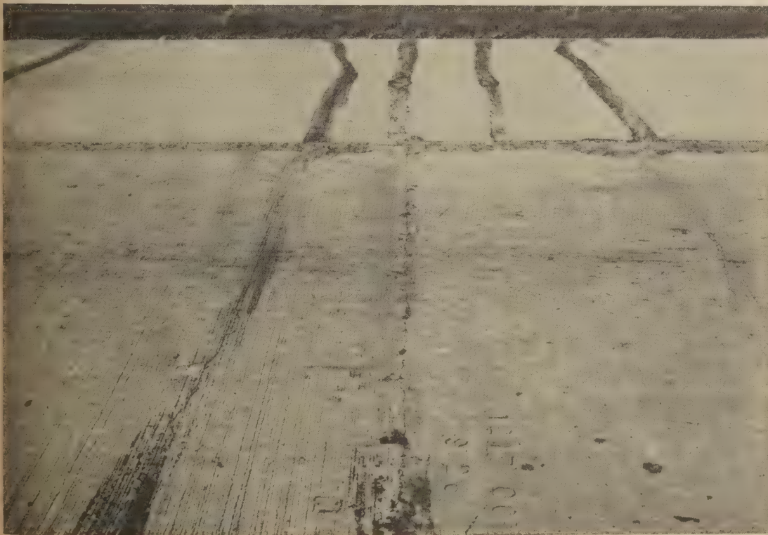
Figure 13.—Condition after 15½ years of a construction joint in the central portion of a section reinforced with heavy steel bars. Reinforcement was continuous through the joint.
