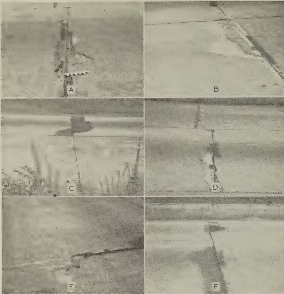
Figure 11.—Spalling at joints occurred principally in the vicinity of Frankfurt.
