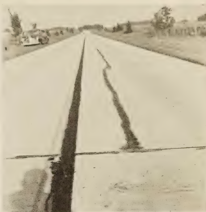
FIGURE 8.—LONGITUDINAL CRACKING IN THE OLDER REINFORCED PAVEMENTS WITH DUMMY CENTER JOINT LAID IN INDIANA IN 1937 (74-E).
