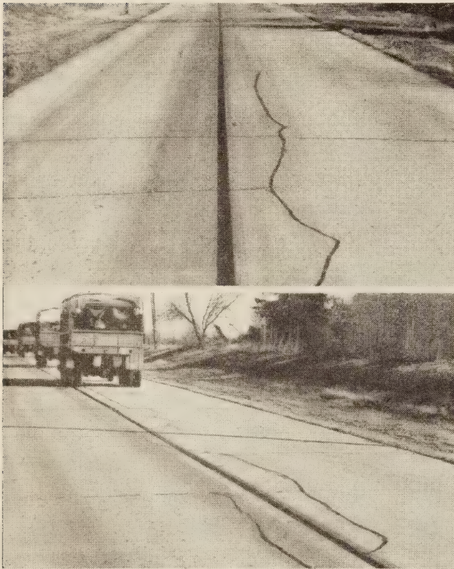
FIGURE 11.—LONGITUDINAL CRACKING IN NEBRASKA PAVEMENTS WITH DUMMY CENTER JOINT, LAID IN 1935-36.
