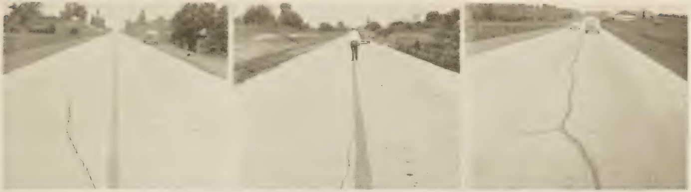
FIGURE 3.—TYPICAL LONGITUDINAL CRACKS IN THE 1942 KENTUCKY PAVEMENTS.
