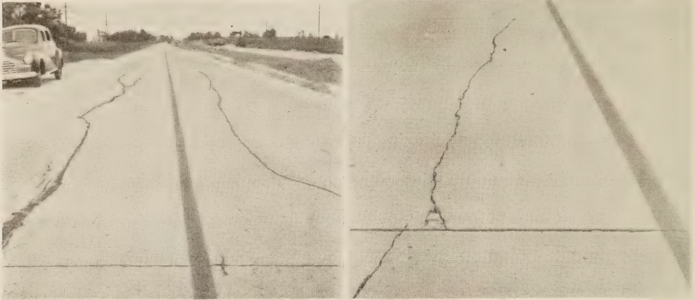
FIGURE 5.—TYPICAL LONGITUDINAL CRACKS OBSERVED IN 1943 IN INDIANA PAVEMENT SN-FA 13-B (2).
