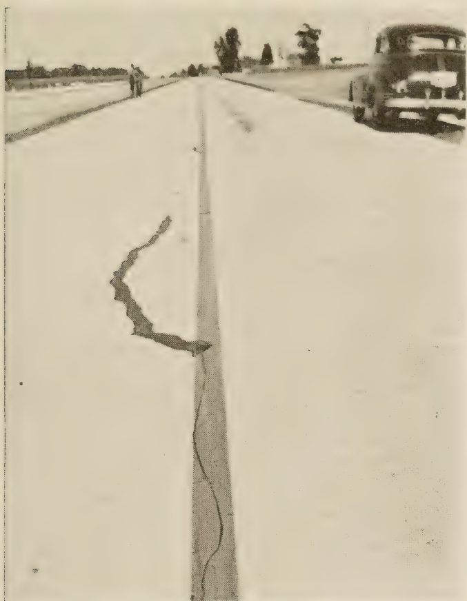
FIGURE 7.—TYPICAL LONGITUDINAL CRACKS IN INDIANA PAVEMENT SN-FA 74 A (2), A (3), B (5).
