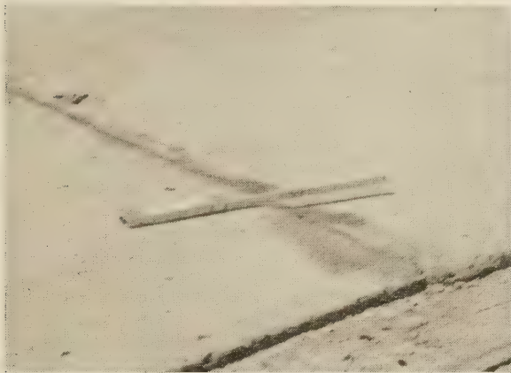
FIGURE 6.—EXPANSION JOINT FAULTED APPROXIMATELY 1 INCH WITH THE SLAB BEYOND THE JOINT DOWN.
