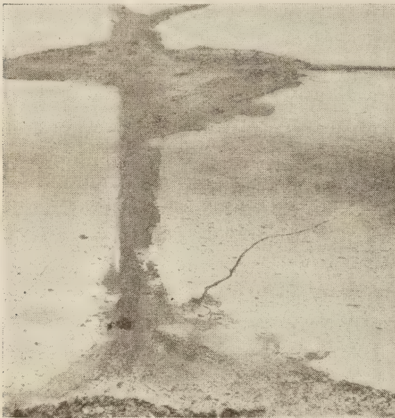
FIGURE 19.—SCALING IN CORNERS FORMED BY EXPANSION JOINT.
