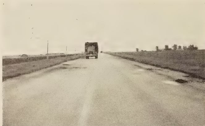
Figure 14.—A BITUMINOUS SURFACE THAT FAILED AFTER 1 YEAR OF SERVICE.
