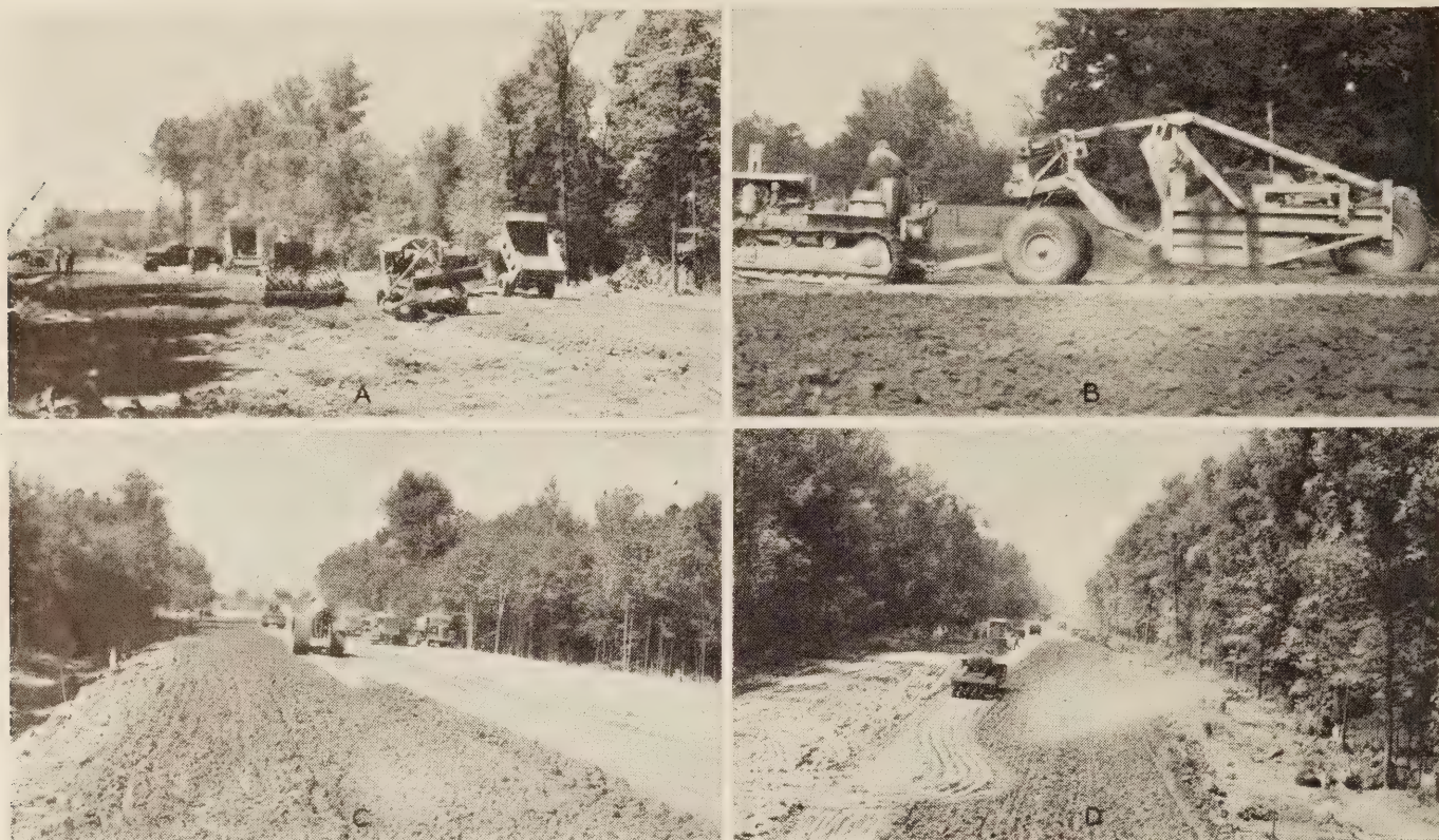
FIGURE 20.—CONSTRUCTION OF GRADE IN INDIANA SHOWING: (A) FOUNDATION LAYER OVER SOFT SOIL; (B) LARGE SCRAPER PLACING FILL MATERIAL ON SECTION 1; (C) COMPACTING WITH THREE-WHEEL 10-TON ROLLER; AND (D) COMPACTING WITH PNEUMATIC TIRE ROLLER.
