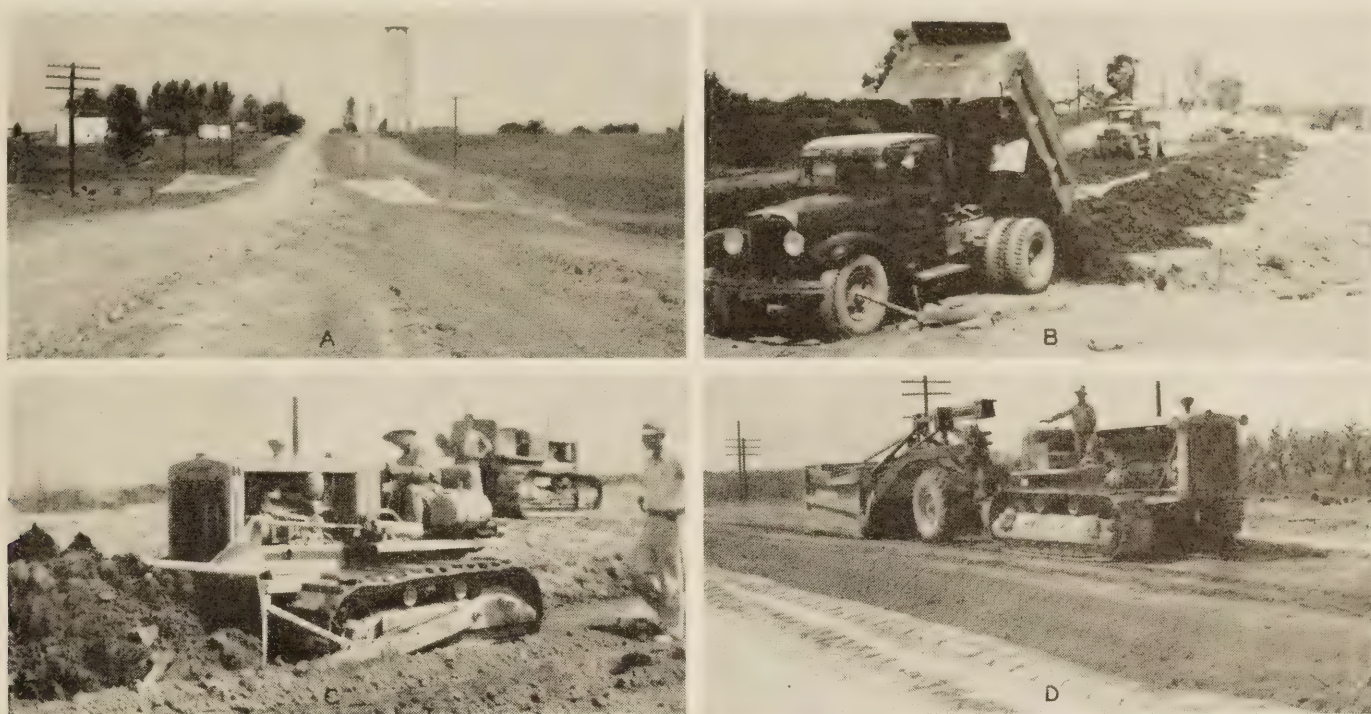
FIGURE 21.—TEST SECTION 4 IN OHIO SHOWING: (A) OLD FILL CLEARED AND READY FOR WIDENING AND RAISING OF THE GRADE; (B) HAULING WITH DUMP TRUCKS; (C) SPREADING WITH BULLDOZER; AND (D) HAULING AND SPREADING WITH SCRAPER.
