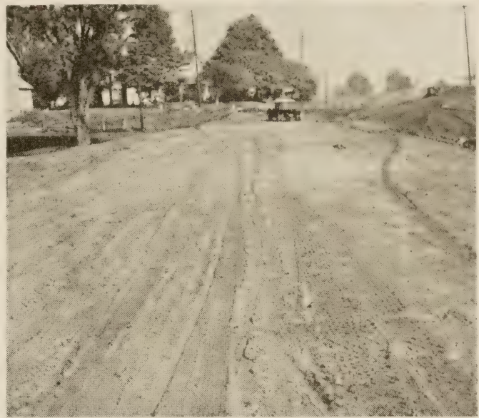
FIGURE 28.—COMPACTED FILL IN OHIO AFTER RAIN. THE SURFACE IS SLICK AND SLUSHY BUT NOT RUTTED.
