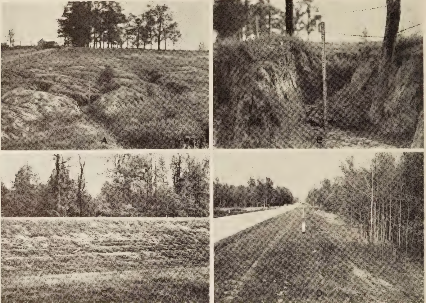
FIGURE 29.—EROSION IN INDIANA (A) OF THE SHEET AND GULLY TYPE IN BORROW PIT A, (B) CHANNELS DRAIN INTO OUTLET IN BORROW PIT A, (C) IN FILL SLOPE BEFORE GOOD COVER OF LESPEDEZA WAS ESTABLISHED, AND (D) TYPICAL CONDITION OF SHOULDERS AND SLOPES ON ENTIRE PROJECT.
