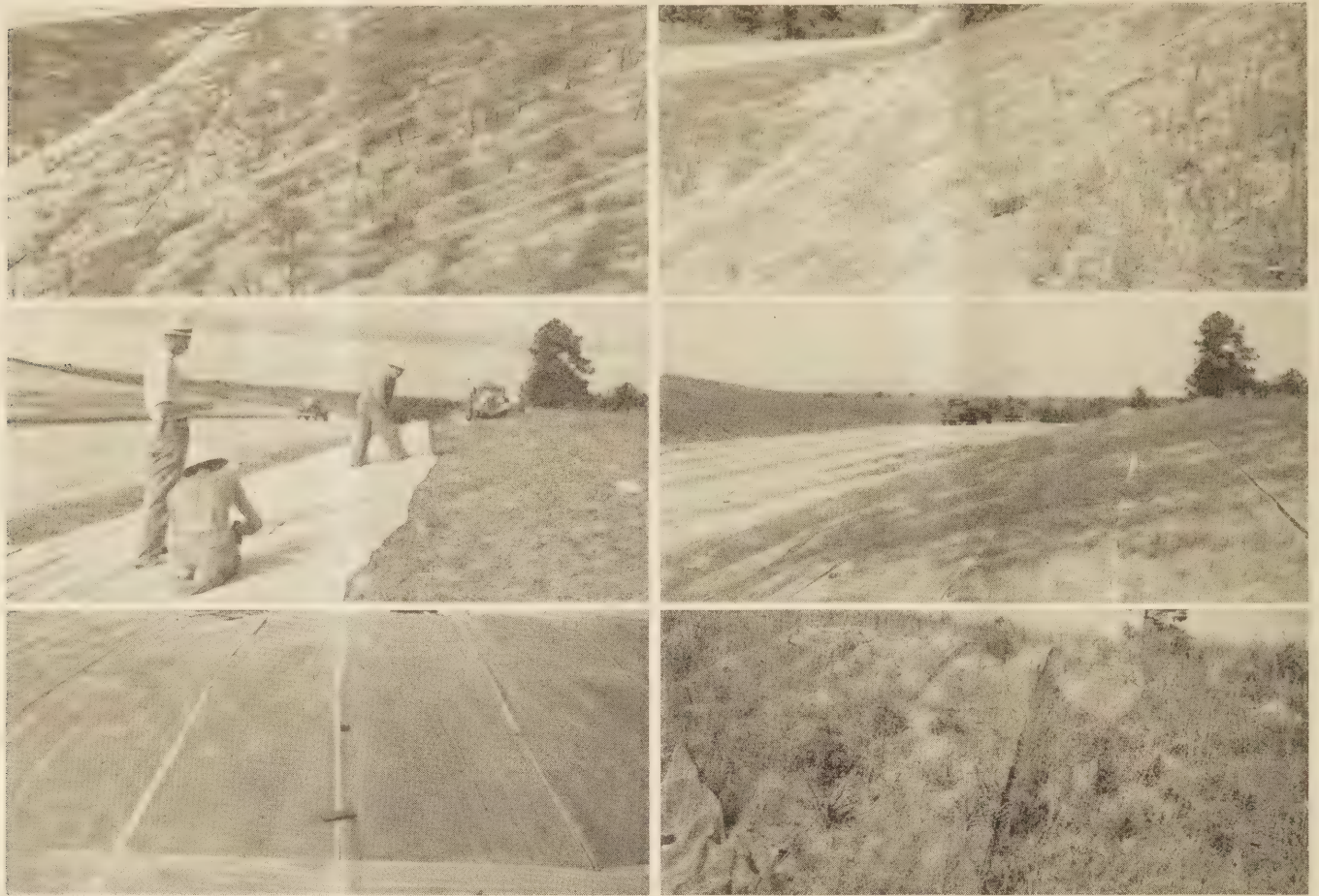
FIGURE 2.—LEFT, APPEARANCE OF PORTIONS OF SECTIONS B (TOP), C (MIDDLE), AND D (BOTTOM) DURING OR SOON AFTER PLACING OF FABRIC; RIGHT, APPEARANCE OF THE SAME RESPECTIVE PORTIONS AFTER ONE GROWING SEASON.
