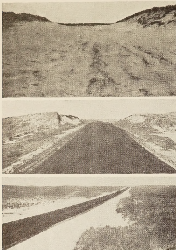
FIGURE 3.—A PORTION OF SECTION 6B BEFORE, AFTER, AND DURING CONSTRUCTION. A, THIS PORTION OF THE ROAD HAD TO BE RESTORED TO GRADE TWICE BEFORE THE SURFACE WAS MIXED. B, SAME AREA SHOWN IN A AFTER THE MAT WAS COMPLETED AND THE SHOULDERS AND SLOPES HAD BEEN SEEDED AND COVERED WITH HAY TO PREVENT WATER AND WIND EROSION. C, CONSTRUCTING THE MAT THROUGH TYPICAL SAND-HILL COUNTRY.
