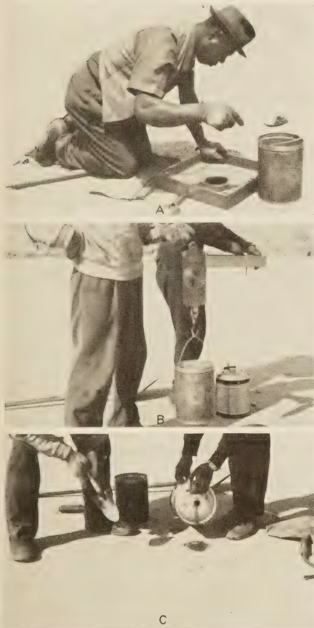
FIGURE 23.—THREE STEPS IN MAKING A DENSITY TEST: A, REMOVING LOOSENED BASE COURSE MATERIAL FROM HOLE; B, WEIGHING THE BASE COURSE MATERIAL REMOVED; and C, FILLING HOLE WITH OIL.
