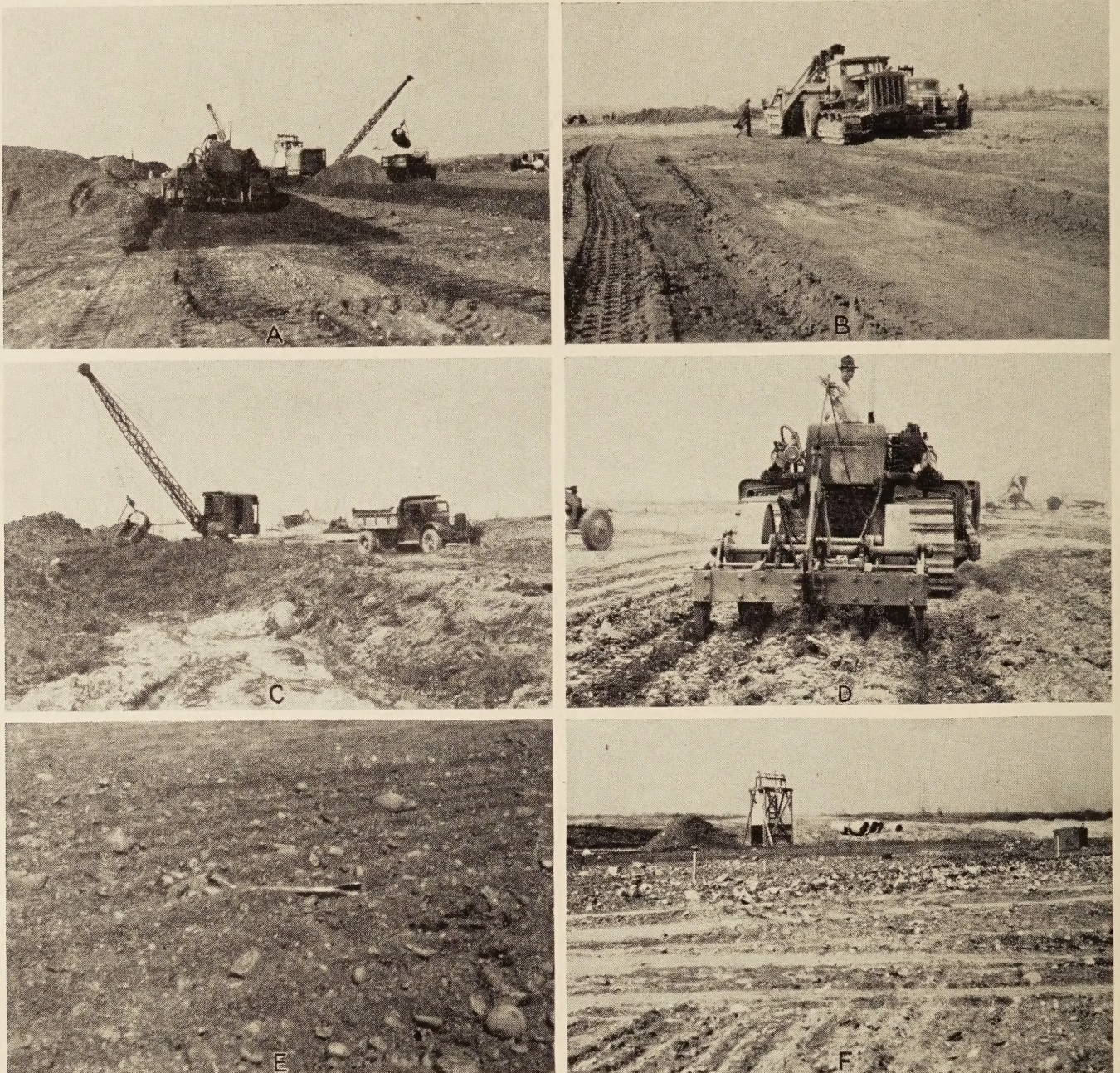
FIGURE 8.—CONSTRUCTION OF RUNWAYS: A, GRADING OPERATIONS; B, THIN LAYERS OF MUCK BEING EXCAVATED BY SCRAPER; C, DEEP MUCK BED BEING EXCAVATED BY DRAGLINE; D, SCARIFYING MATERIAL WITH HEAVY-DUTY ROOTER; E, OVERSIZE STONE BROUGHT TO SURFACE BY SCARIFYING; AND F, OVERSIZE STONE IN EXCESSIVE AMOUNTS GENERALLY ENCOUNTERED AT RUNWAY INTERSECTIONS.
