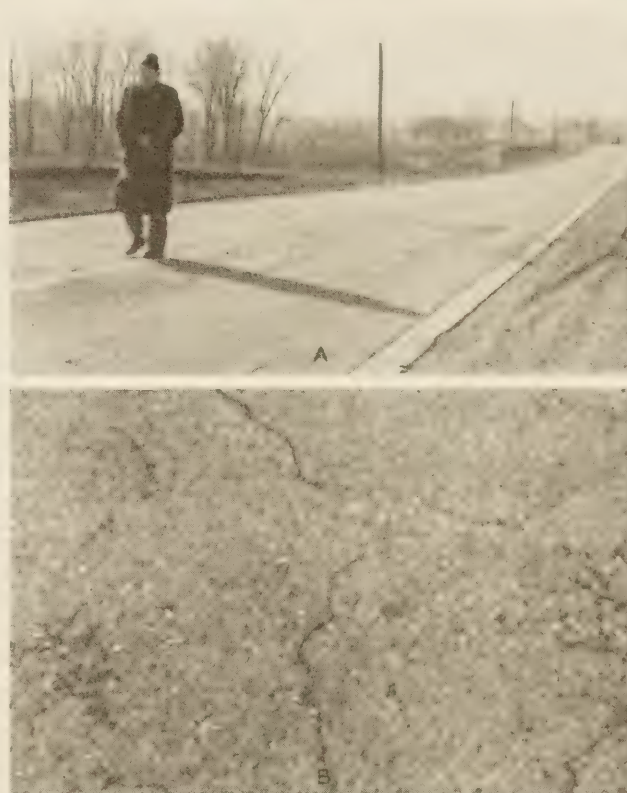
FIGURE 2.—A, GENERAL VIEW, AND B, SURFACE DETAIL OF A PAVEMENT THAT WAS RATED VERY POOR. NOTE THE SPALLING ALONG THE CRACKS AND THE RAVELED CONDITION OVER A LARGE PORTION OF THE PAVEMENT. SAMPLE S B WAS TAKEN AT THIS LOCATION. THE PATCHED SAMPLE HOLE CAN BE SEEN IN THE RIGHT CENTER OF THE UPPER PICTURE.
