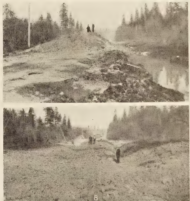
FIGURE 8.—A, OLD ROAD LOADED WITH BORROW MATERIAL BEFORE UNDERFILL BLASTING; B, THE SAME SECTION OF ROAD SHOWN IN A AFTER BLASTING. THE FILL MASS SETTLED APPROXIMATELY 15 FEET. NOTE THE SWAMP MUCK PUSHED OUT ON EACH SIDE.
