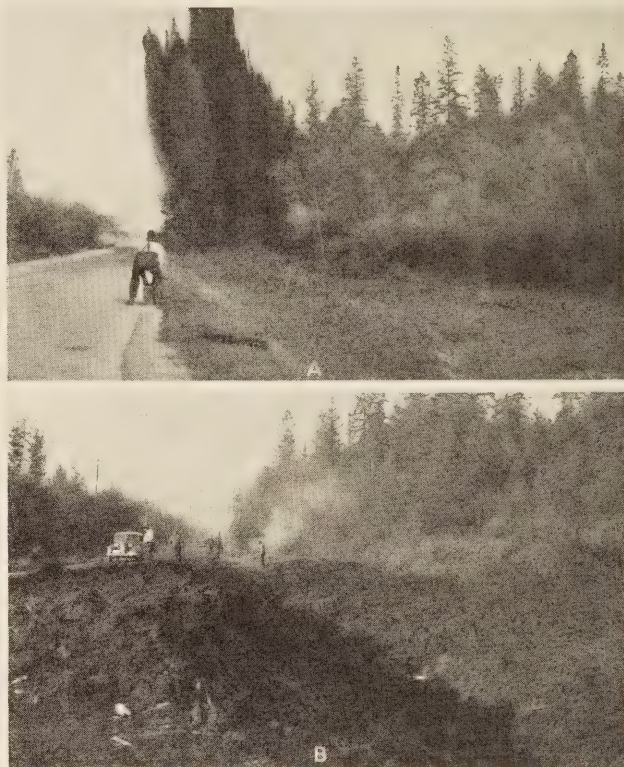
FIGURE 6.—A, BLAST IN WHICH A DELAY CAP WAS USED TO FIRE THE INSIDE ROW OF CHARGES. B, RELIEF DITCH OBTAINED BY BLASTING THE SWAMP MAT.
