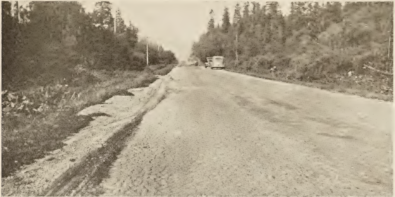
FIGURE 1.—EXISTING ROAD PRIOR TO RECONSTRUCTION. PICTURE TAKEN AT STATION 235, SHOWING CRACKS CAUSED BY UNSTABLE SUBGRADE.
