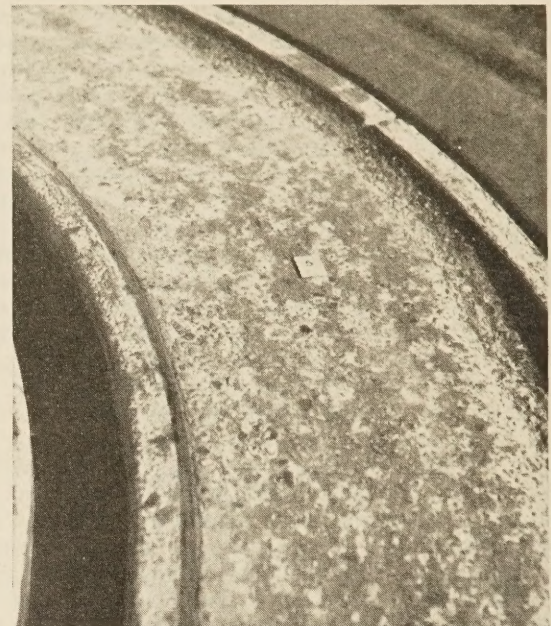
FIGURE 7.—SECTION 5 OF TRACK 2 AT 184,000 WHEEL-TRIPS, JUST BEFORE THE FIRST SPRINKLING. SOME RAVELING HAD DEVELOPED, PARTICULARLY ALONG THE EDGES.
