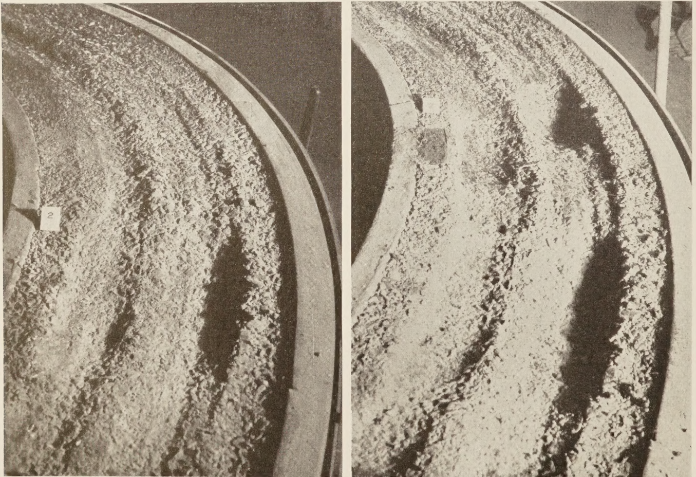
FIGURE 5.—APPEARANCE OF SECTION 2 OF SERIES 2: LEFT, AFTER 205,000 WHEEL-TRIPS, WHEN FAILURE BECAME EVIDENT (NOTE THAT THE SURFACE TREATMENT WAS COMPLETELY SHEARED THROUGH AT THE DEPRESSION IN THE OUTSIDE RUT); RIGHT, AFTER 255,000 WHEEL-TRIPS.
