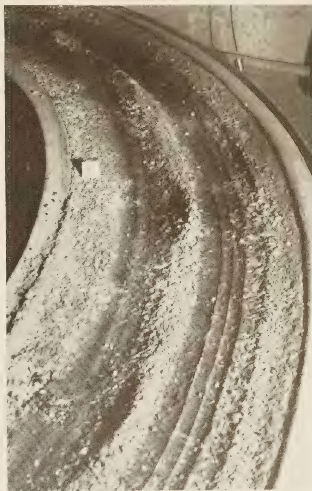
FIGURE 6.—APPEARANCE OF SECTION 6 OF SERIES 2 AFTER 255,000 WHEEL-TRIPS OF TRAFFIC. FAILURE IS INDICATED BY THE GENERAL ROUGHNESS, RUTTING, AND BREAKING OF THE SURFACE-TREATMENT.
