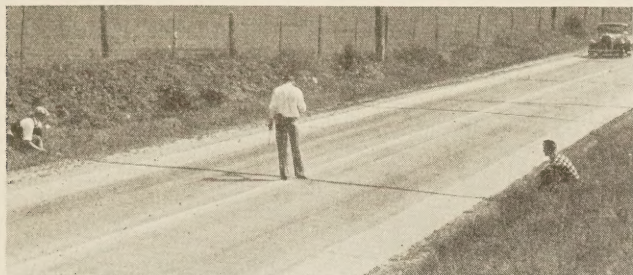
FIGURE 2.—DETECTOR TUBE BEING INSTALLED. THE TUBE IS CENTERED AND THE ENDS FASTENED BY SPIKES.
