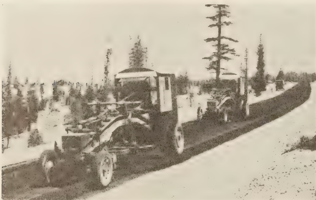
MIXING OIL-TREATED GRAVEL IN THE CONSTRUCTION OF A FLEXIBLE-TYPE ROAD SURFACE. THE RESISTANCE THAT THIS TYPE OF SURFACE OFFERS TO DEFORMATION UNDER LOAD DEPENDS ESSENTIALLY UPON THE DEGREE OF COHESION AND INTERNAL FRICTION IT POSSESSES.
