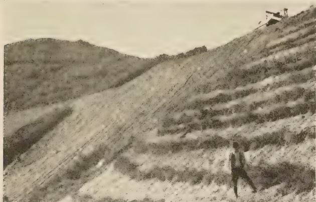
FIGURE 6.—APPEARANCES OF PROTECTED AND UNPROTECTED FILL SLOPES AFTER A HEAVY RAIN.
