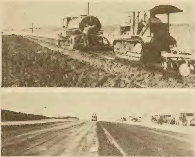
FIGURE 21.—UPPER; APPLYING BITUMINOUS EMULSION AND MIXING WITH A DISK HARROW. LOWER; ROLLING A BASE COURSE STABILIZED WITH BITUMINOUS EMULSION.
