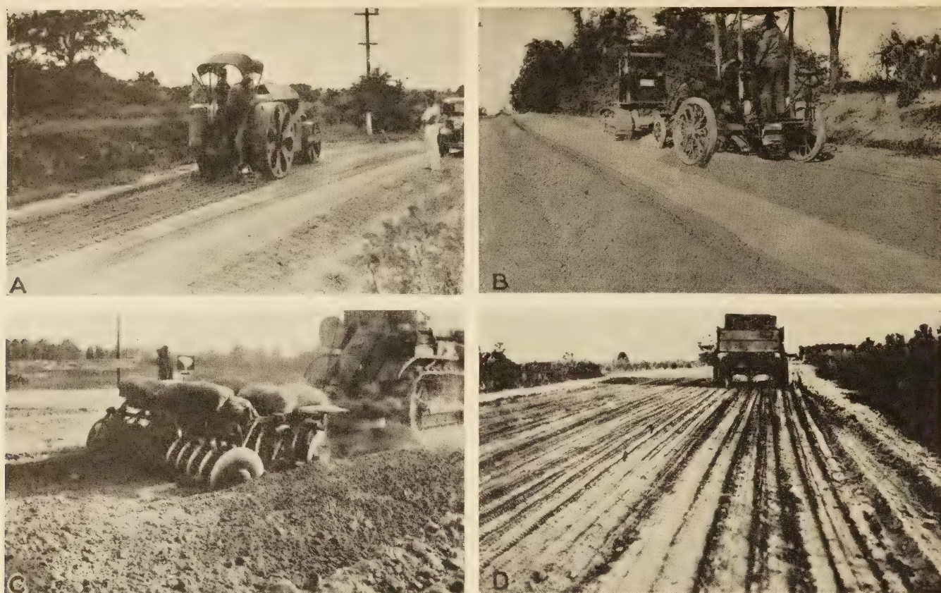
FIGURE 20.—STEPS IN THE CONSTRUCTION OF STABILIZED SOIL ROADS. A, SCARIFYING A GRAVEL ROAD; THE LOOSENING AGGREGATE WILL BE USED IN THE STABILIZED MIXTURE. B, MIXING THE DRY MATERIALS WITH A BLADE GRADER. C, MIXING THE DRY MATERIALS FOR A CEMENT-TREATED ROAD WITH A DISK HARROW. D, COMPACTING THE WET MATERIALS ON A CEMENT-TREATED ROAD.
