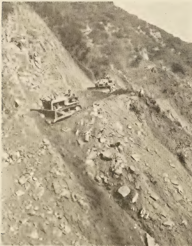
BULLDOZERS CAN OFTEN BE USED IN OPENING THE CUT AND PREPARING A HAULING ROAD AHEAD OF THE SHOVEL.
