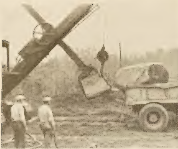
LARGE BOULDERS ARE HARD ON EQUIPMENT AND DECREASE THE RATE OF PRODUCTION. THEY SHOULD BE REDUCED BY BLASTING.
