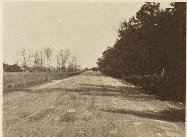
FIGURE 3.—FAILURE OF THE HEAVY NONSKID TREATMENT ON SECTION 8
