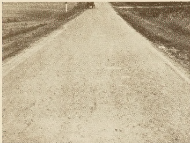
FIGURE 7.—TYPICAL CONDITION OF THE PORTION OF SECTION 10 WHICH WAS NEVER RE-TREATED
