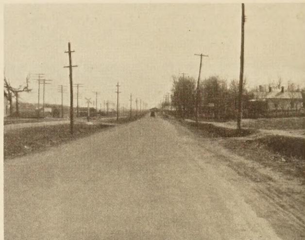
FIGURE 8.—VIEW OF THE SOUTH END OF SECTION 11, SHOWING THE EXCELLENT CONDITION OF THE PORTION NEVER RE-TREATED
