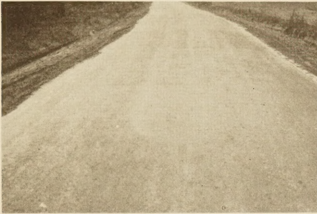
FIGURE 4.—PORTION OF SECTION 8 NEVER RE-TREATED AFTER CONSTRUCTION, PHOTOGRAPHED IN APRIL, 1930
