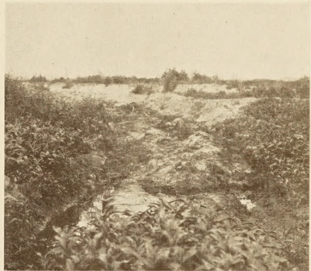
FIGURE 2.—WET AREA AT STATION 20+00. POWER SHOVEL WAS STUCK AT THIS POINT
