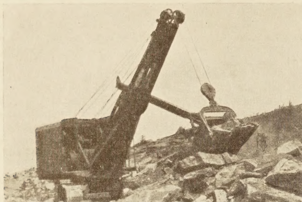
FIGURE 7.—SHALLOW CUTS IN HARD ROCK ALWAYS PROVE EXPENSIVE. ALTHOUGH THE CONTRACTOR SPENT $2 PER CUBIC YARD ON DRILLING AND BLASTING IN THIS CUT (MOSTLY 2 TO 4 FEET DEEP), THE ROCK WAS STILL SO POORLY BROKEN THAT THE COST OF GETTING IT INTO THE FILL ADDED OVER ANOTHER DOLLAR
