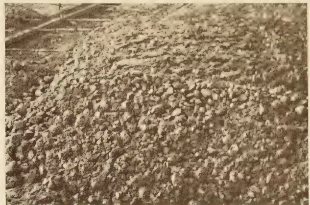
FIGURE 5.—THE LAST CUBIC FOOT OF CONCRETE DISCHARGED FROM ANY MAKE OF MIXER HAS A PREDOMINANCE OF COARSE AGGREGATE. THE DESIGN OF MIXER SPREADER-BUCKETS ALSO AFFECTS SEGREGATION. THE RESULTS OF THESE TWO EFFECTS CAUSED A BATCH TO APPEAR AS SHOWN
