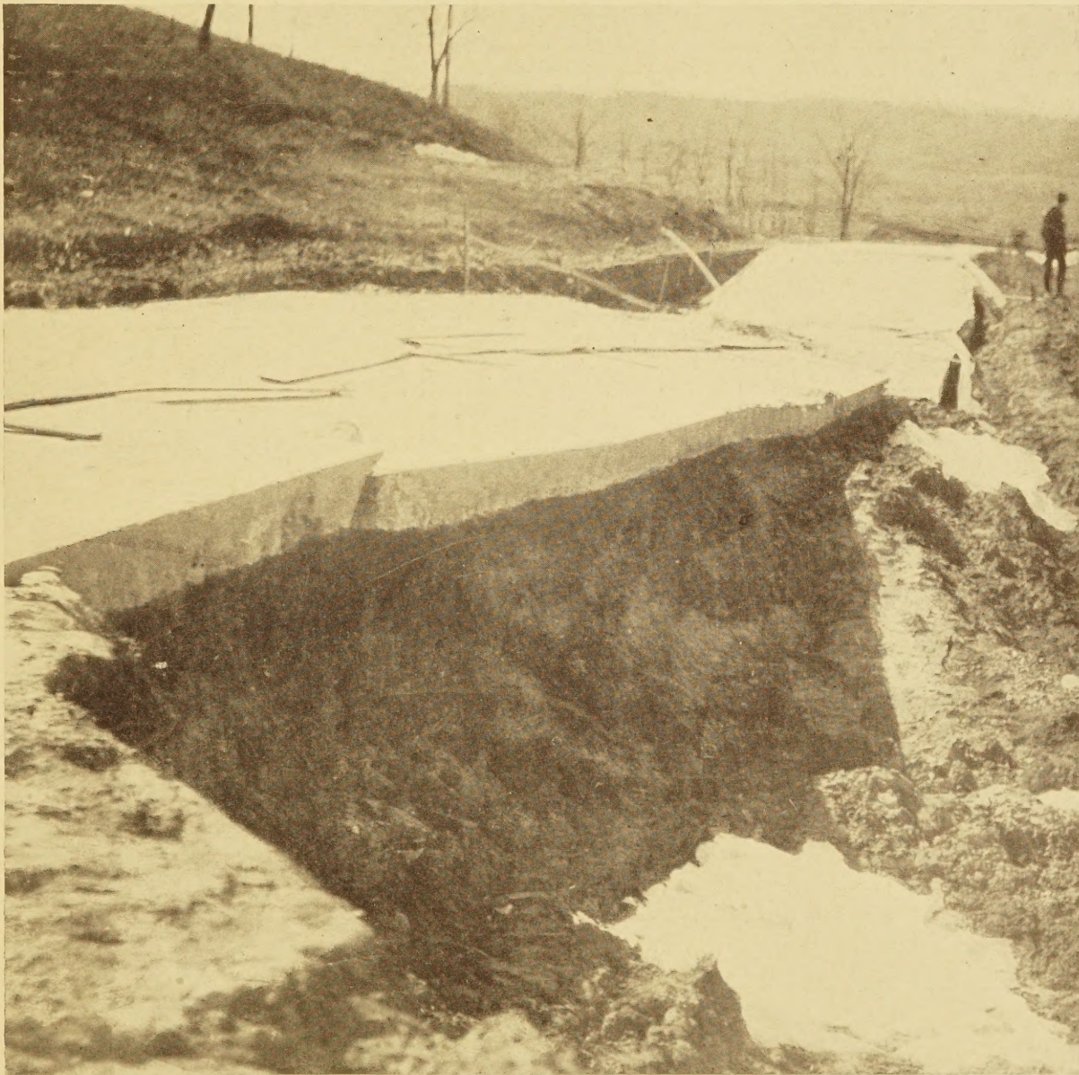
PAVEMENT FAILURE CAUSED BY SLIDE IN SIDE FILL
