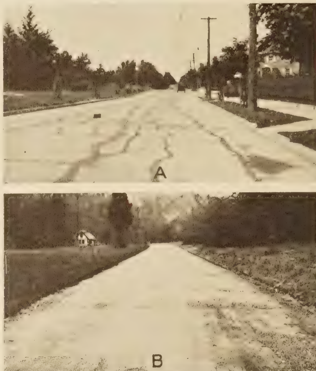
FIGURE 15.—DETRIMENTAL EFFECTS OF ELASTICITY OF SUBGRADE SOIL. A.—TYPE OF CRACKING LIKELY TO OCCUR IN PAVEMENTS LAID ON IMPROPERLY PREPARED ELASTIC SUBGRADES. NOTE CRACKS REFLECTING RUTS IN SUBGRADE. B.—ALLIGATOR HIDE CRACKING IN MACADAM ROAD SURFACE
