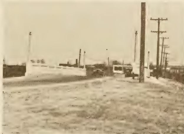
FIGURE 17.—SETTLEMENT OF ROAD AT BRIDGE APPROACH DUE PRIMARILY TO THE CONSOLIDATION OF THE THOROUGHLY SATURATED UNDERSOIL
