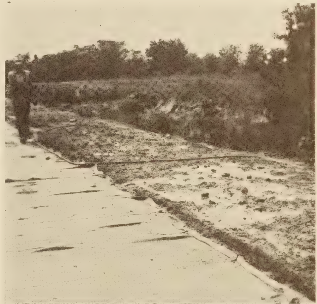
WET BURLAP ON ONE SIDE OF LONGITUDINAL JOINT, EARTH AND WATER CURE ON OTHER SIDE
