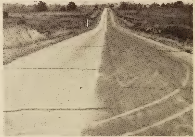
BITUMINOUS-CURED AND STANDARD-CURED SECTIONS AFTER FORMATION OF CRACKS. NOTE CRACK SPACING ON EITHER SIDE OF LONGITUDINAL JOINT
