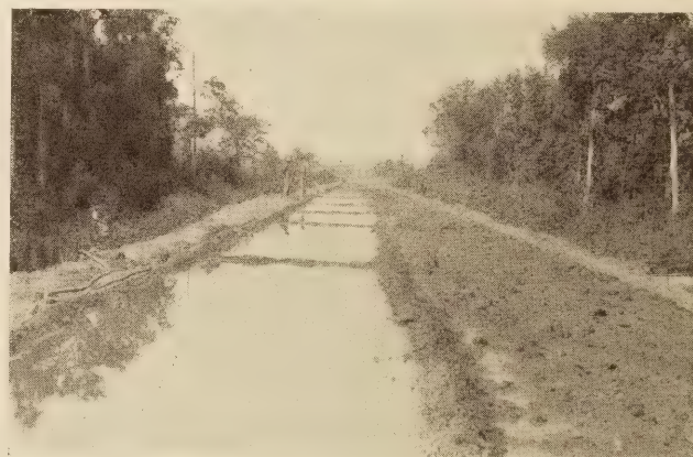
PONDING ON ONE SIDE, STANDARD EARTH AND WATER CURE ON THE OTHER
