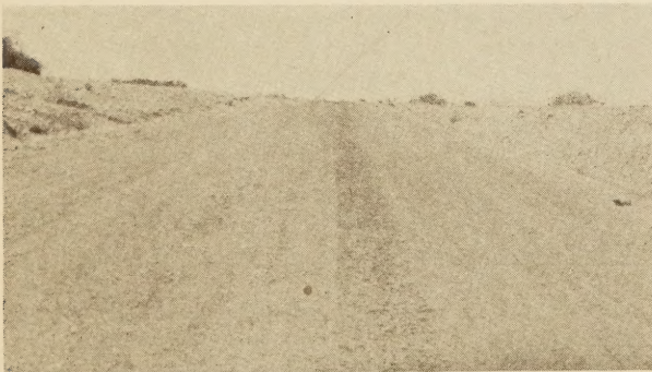
A THREE-INCH OIL-MIX ROAD IN ARIZONA. EARLY FAILURES OCCURRED BECAUSE THE AGGREGATE CONTAINED CALICHE
