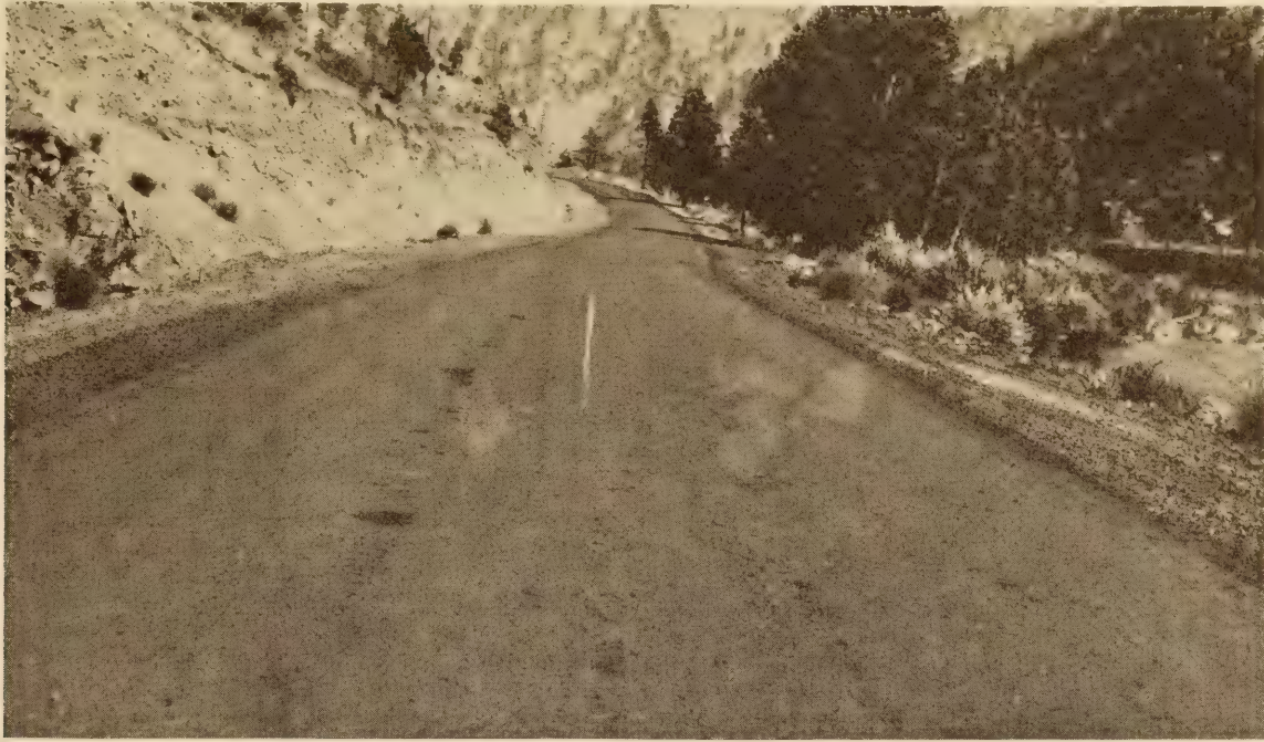
EARLY RAVELING DEVELOPS WHEN INSUFFICIENT OIL IS USED IN CONSTRUCTION. THIS MIX CONTAINS ABOUT 25 PER CENT MORE OIL THAN CALLED FOR BY MCKESSON AND FRICKSTAD FORMULA
