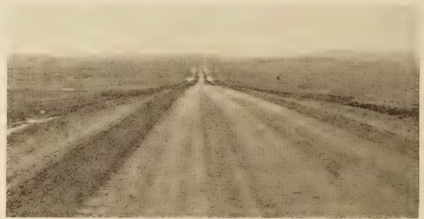
LIGHT-OIL-MIXED SURFACE RAPIDLY FAILING ON ACCOUNT OF INSUFFICIENT OIL. NOTE COARSE AGGREGATE THROWN TO THE EDGES
