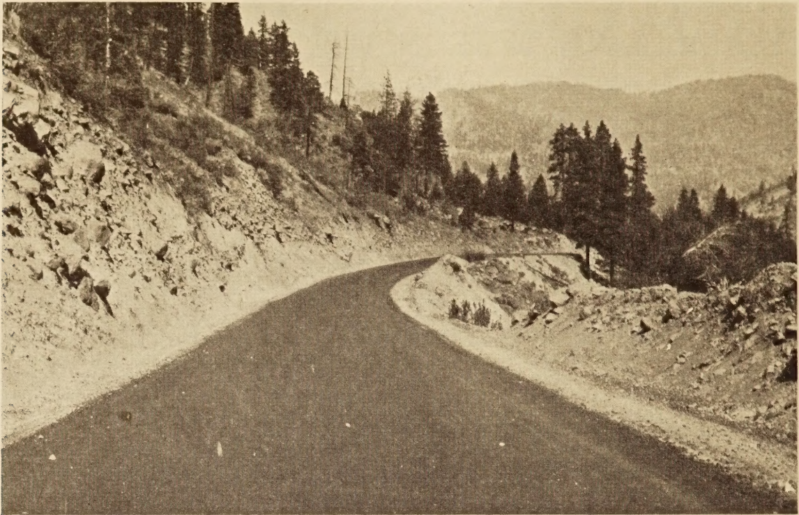
MIXED-IN-PLACE SURFACE CONSTRUCTED OF CRUSHED STONE AND 94 PER CENT ROAD OIL CUT BACK WITH KEROSENE
