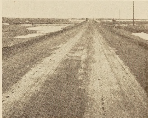
TYPICAL APPEARANCE OF BLEEDING ON A LIGHT OIL-MIXED SURFACE CAUSED NOT BY EXCESS OIL BUT BY MOISTURE AND OIL RISING TO THE SURFACE
