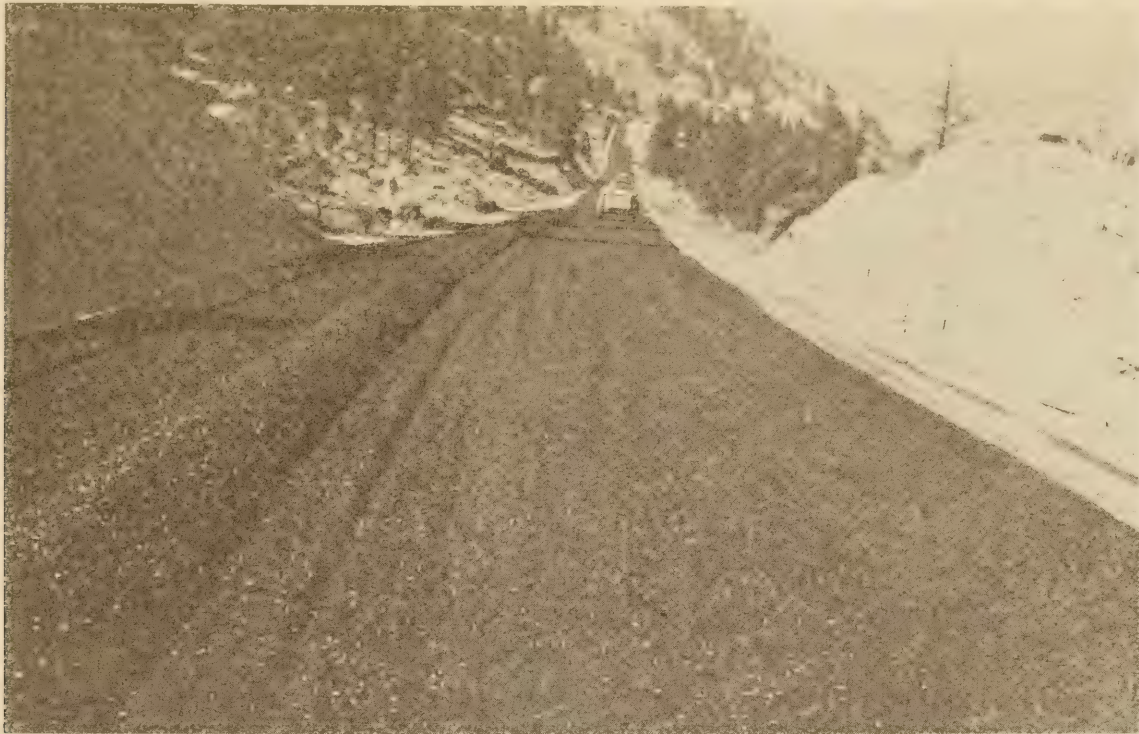
100 TO 120 PENETRATION ASPHALT CUT BACK WITH KEROSENE. SMOOTHING OF THE MIX PRIOR TO COMPACTION
