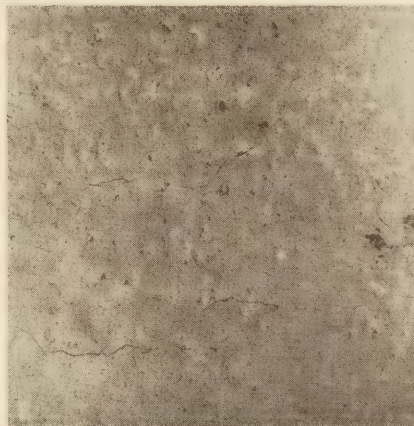
Section 15, dry subgrade, 2 per cent calcium chloride admixture with no surface curing treatment, note local shrinkage and crazing cracks
