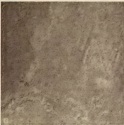
Section 28, wet subgrade, wet burlap for 24 hours, then an application of sodium silicate (4 parts sodium silicate, 42 Baumé to 1 part water), imprint of burlap evident and surface free from local shrinkage cracks
