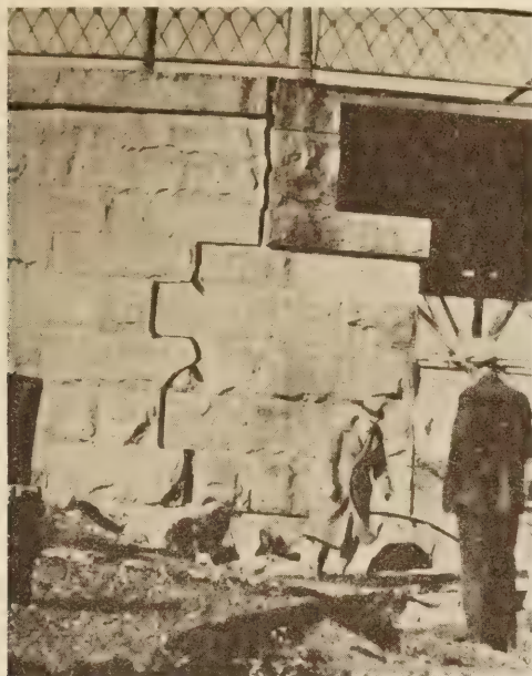
FIGURE 19.—CRACK SEPARATING ABUTMENT FROM WING WALL. HIGHWAY BRIDGE CROSSING MERRIMAC RIVER, MASS.
