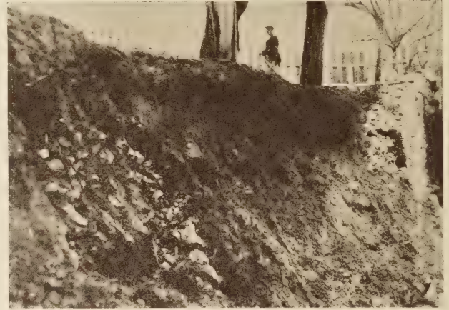
FIGURE 18.—CONDITION OF BACK FILL AFTER FAILURE OF RETAINING WALL
