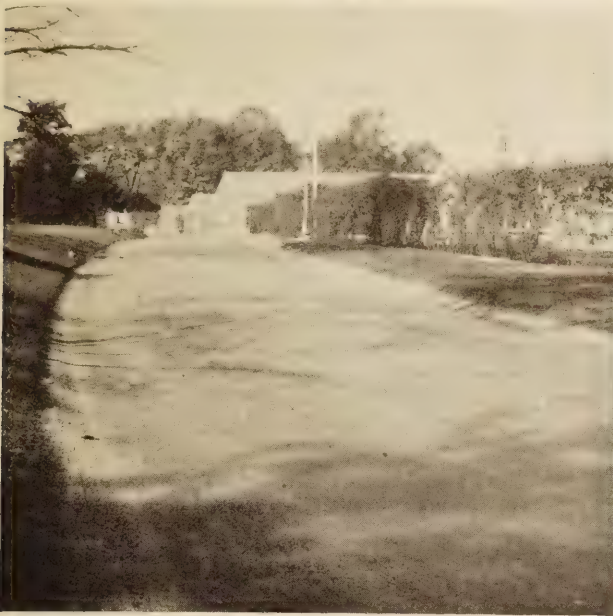
FIGURE 6.—PRESENT APPEARANCE OF THE EAST END OF SECTION 2. ALTHOUGH LYING IN A CUT THE BITUMINOUS GUTTERS AND NATURAL SLOPE AFFORD AMPLE DRAINAGE
