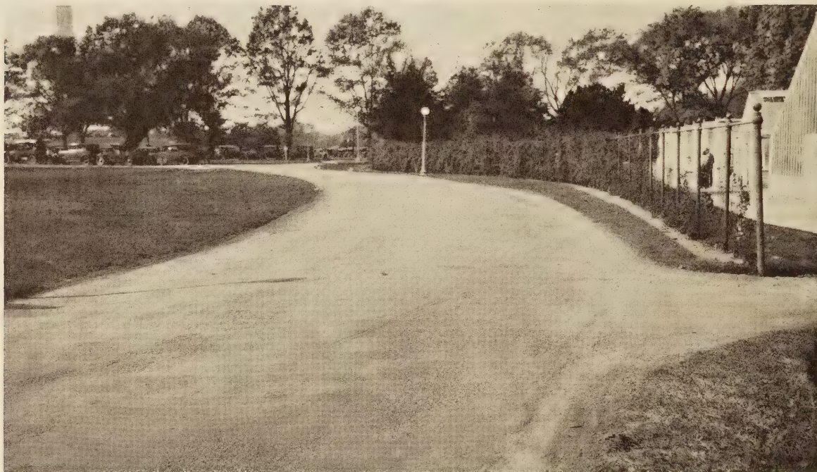
FIGURE 5.—PRESENT CONDITION OF THE CENTRAL PORTION OF SECTION 2. NOTE HEAVY PATCHING AND SHOWING OF THE SURFACE MAT ALONG RIGHT SIDE
