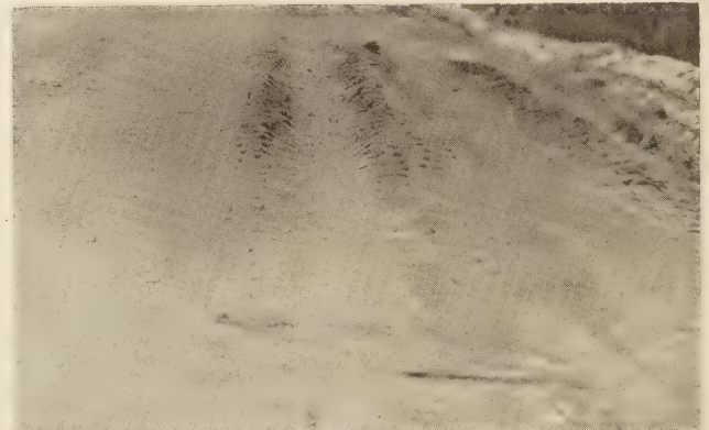
FIGURE 21.—FAILURE OF MACADAM BASE ON A GROUP A-7 SUBGRADE. THE ELASTICITY OF THE SUBGRADE PERMITTED BOND IN THE MACADAM TO BE DESTROYED, AFTER WHICH LATERAL FLOW OCCURRED IN THE SUBGRADE
