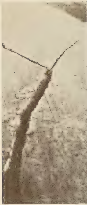
FIGURE 11.—SEPARATION OF SLAB FRAGMENTS DUE TO SUBGRADE CONDITIONS
