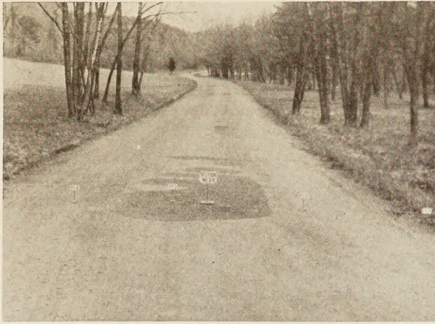
FIGURE 4.—FAILURE LOCALIZED TO SOFT SPOT IN SUBGRADE
