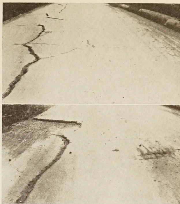
FIGURE 7.—CRACKING ON A FILL MADE WITH CLAY HAVING HIGH SHRINKAGE PROPERTIES
