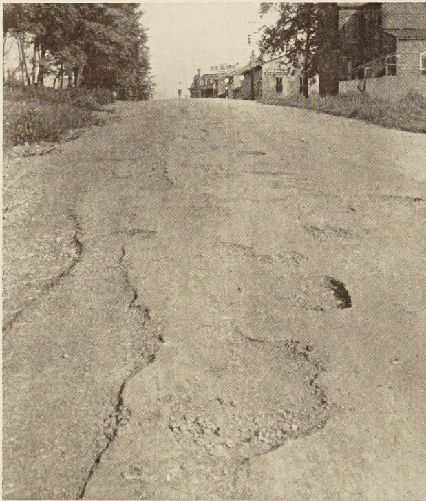
FIGURE 2.—SURFACE FAILURE IN A BITUMINOUS TREATED TRAFFIC-BOUND ROAD
