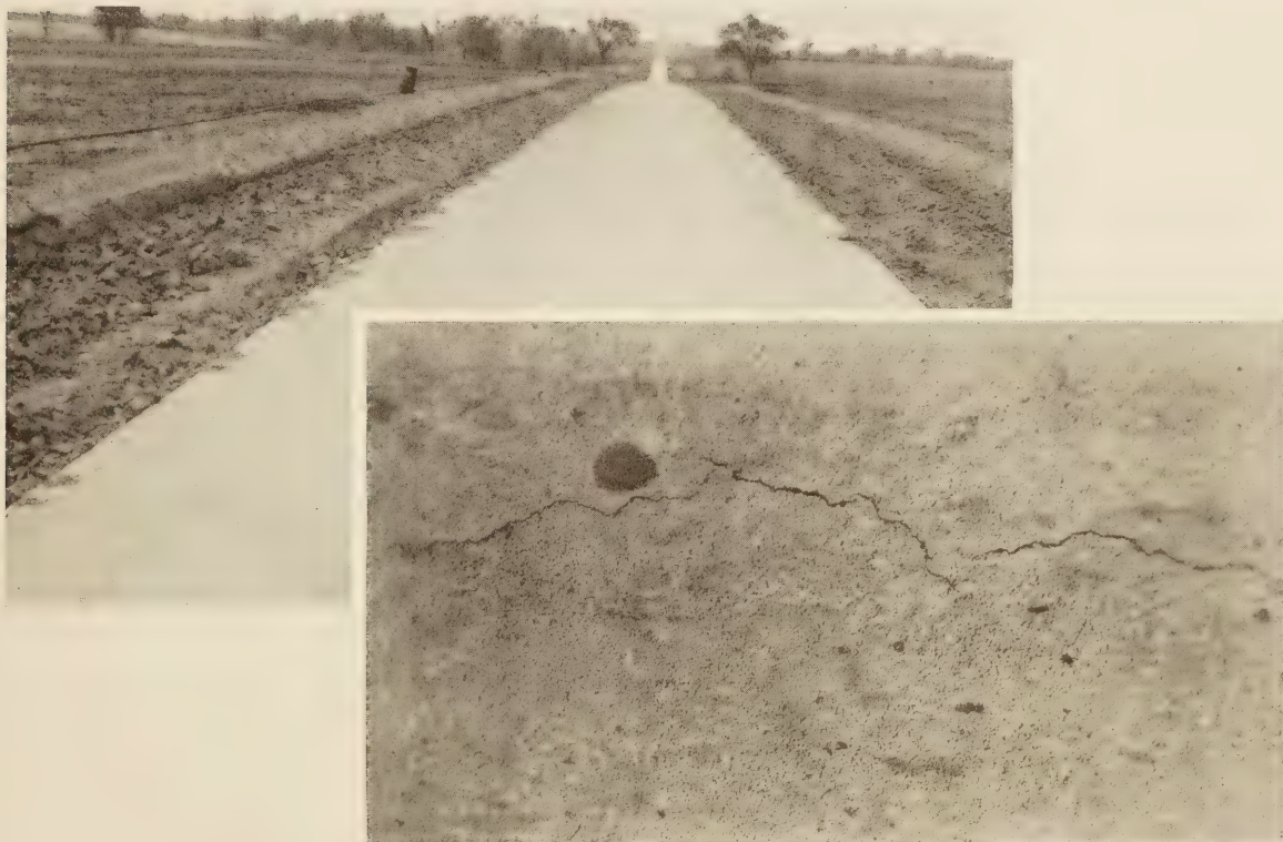
FIGURE 10.—UPPER: CRACKING LOCALIZED IN PORTIONS OF CONCRETE LAID OVER WHEEL PATHS IN SUBGRADE. LOWER: IRREGULAR CRACKING CAUSED BY EXPANSION IN THE SUBGRADE COMBINED POSSIBLY WITH SHRINKAGE IN THE CONCRETE DUE TO LOSS OF WATER FROM THE CONCRETE BEFORE SETTING
