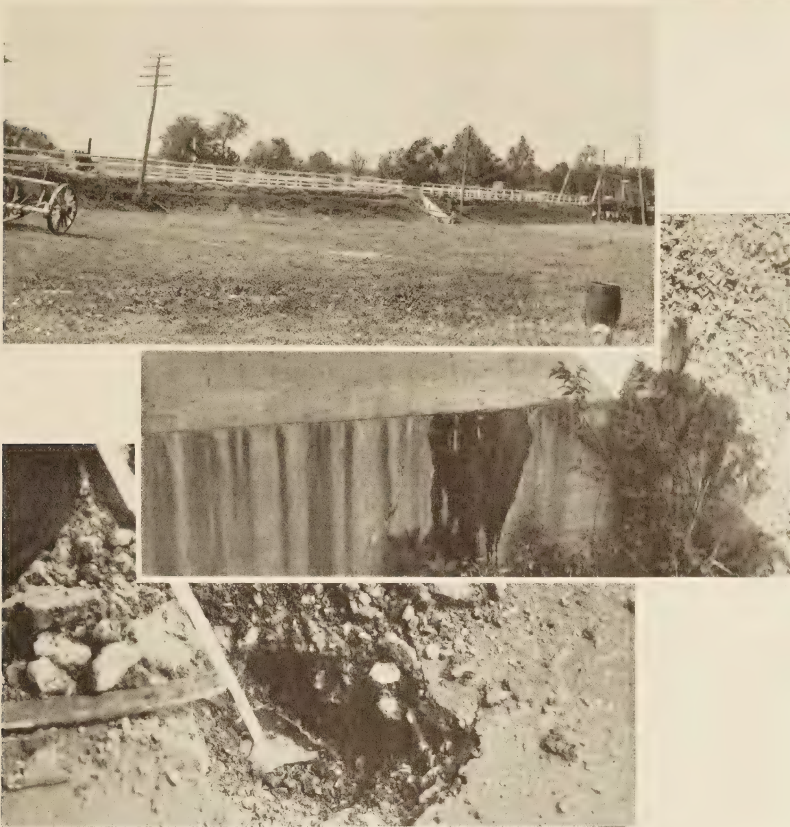
FIGURE 24.—A FILL IN WHICH WATER WAS TRAPPED, WATER SEEPING THROUGH THE ABUTMENT SHOWN IN THE FILL AND WATER SEEPING IN A HOLE CUT IN THE PAVEMENT ON THE FILL
