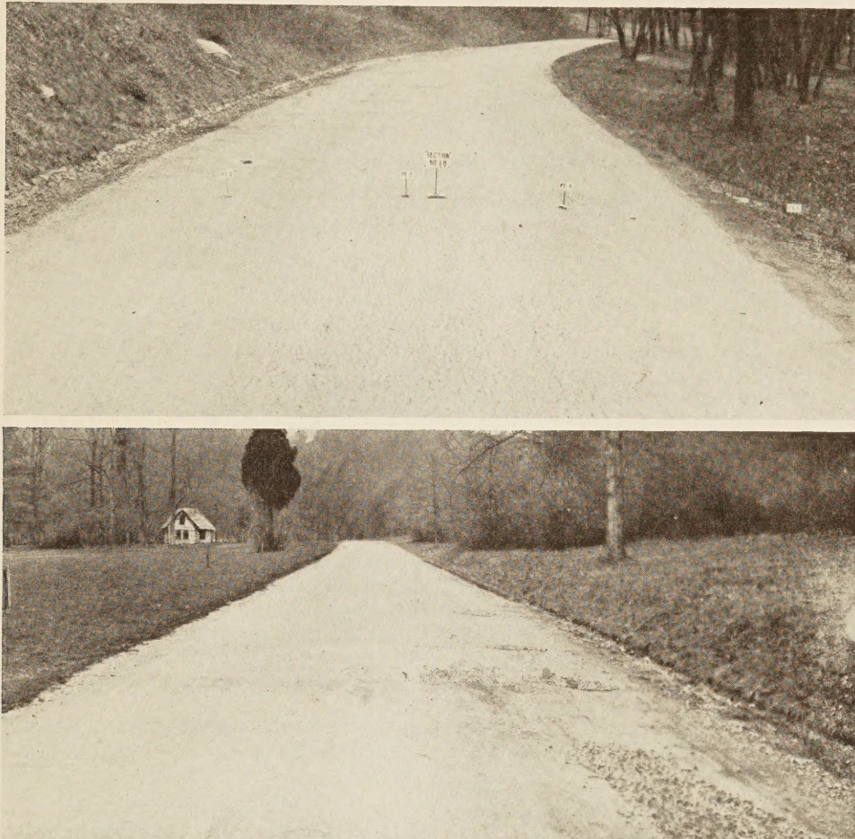
FIGURE 3.—THE UPPER VIEW SHOWS THE BEGINNING OF FAILURE OF MACADAM BASE DUE TO SPONGY SUPPORT, WHILE THE LOWER VIEW SHOWS AN ADVANCED STAGE OF SUCH A FAILURE
