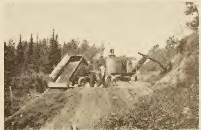
TYPICAL OPERATION WITH LIGHT TRUCKS ON PNEUMATIC TIRES. THE LOWER PICTURE ILLUSTRATES A CASE WHERE SHUTTLING CAN BE PRACTICED TO ADVANTAGE
