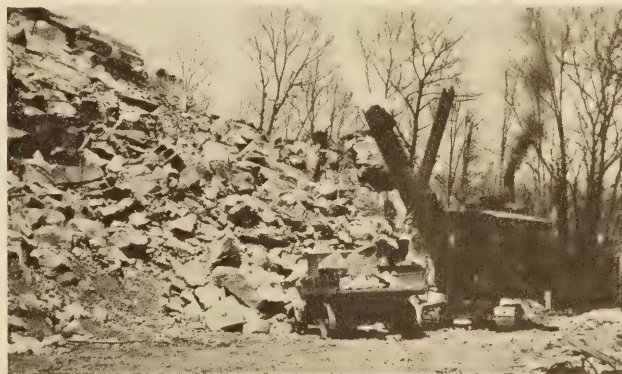
ROADWAY IN GOOD CONDITION AND TRUCK SPOTTED FOR LOADING AT THE SIDE
