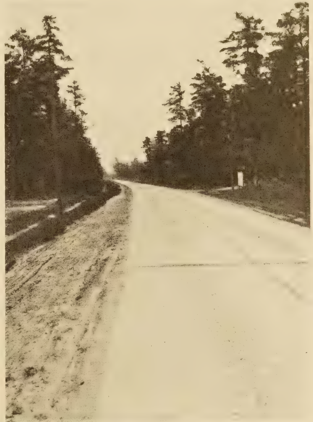
A MODERN CONCRETE PAVEMENT. THE LONGITUDINAL JOINT PREVENTS IRREGULAR LONGITUDINAL CRACKS AND ACTS AS A GUIDE LINE FOR THE TRAFFIC
