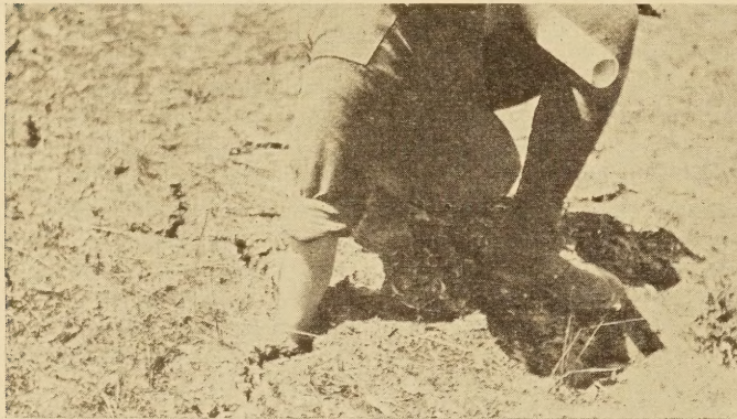
FIG. 1.—Shrinkage cracks in the adobe soil in the open field adjacent to the Pittsburg test road were large enough to admit the arm halfway to the elbow
