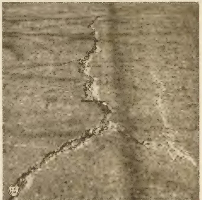
The cracks filled with asphalt have been refilled once and are now badly in need of further attention
