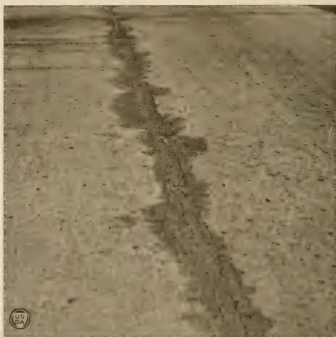
The asphalt filler has flowed out of the joints, forming unsightly black streaks several inches wide
