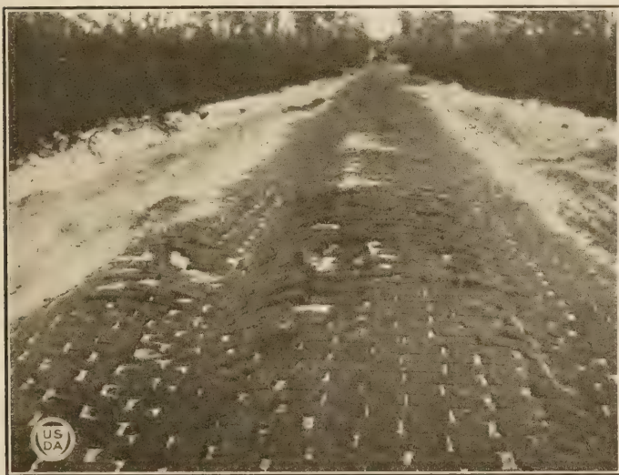
FIG. 14.—Failure of narrow, sand-filled surface between Hastings and Ormond Beach. This is a third-stage pavement.
