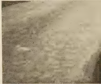
FIG. 18 (RIGHT).—SHOWING HOW EDGES FAILED WHERE WATER STOOD NEAR THE ROAD SURFACE AND SHOULDERS WERE WASHED AWAY.
