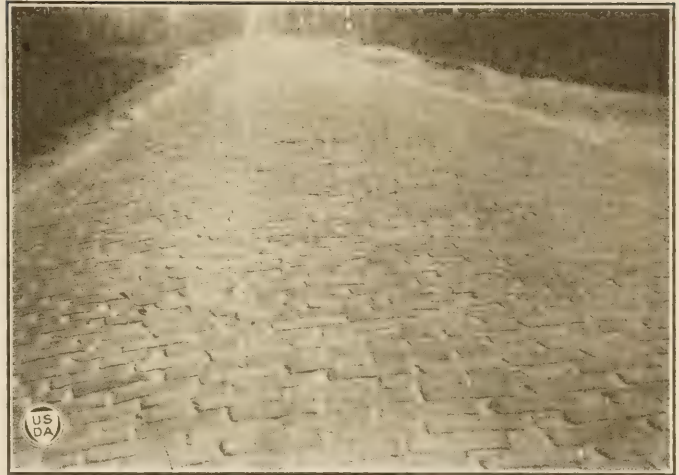
FIG. 12.—Sand-filled brick surface with wood curbs, between Orlando and Sanford. This surface is in the third stage of deterioration. Note the settlement and separation of the brick.
