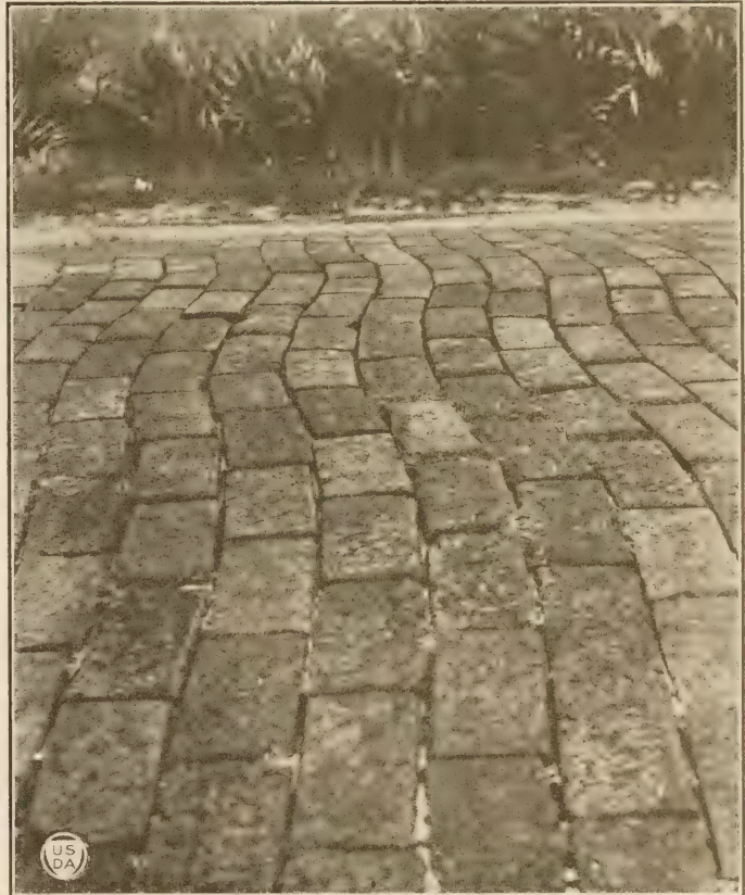
FIG. 9.—Section of sand-filled surface between Jacksonville and Atlantic Beach, showing movement of brick and loss of filler.
