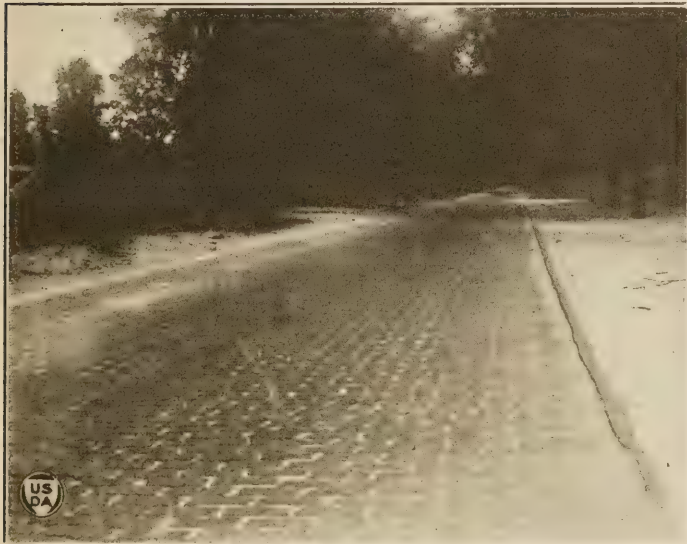
FIG. 8.—Section of sand-filled brick pavement with depressed center—State Route No. 4—north of Jacksonville. Although water has flowed down the middle of this road for 14 years it still presents a good riding surface.
