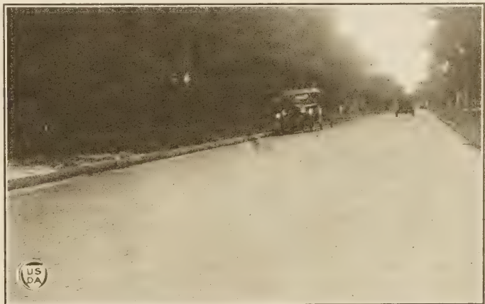
FIG. 3.—Park Avenue, Sanford—A sand-filled pavement in the first stage of deterioration, still giving excellent traffic service.
