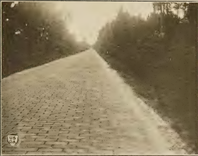
FIG. 7.—Sand-filled brick surface, north of Jacksonville. In the second stage of deterioration but still giving good service.
