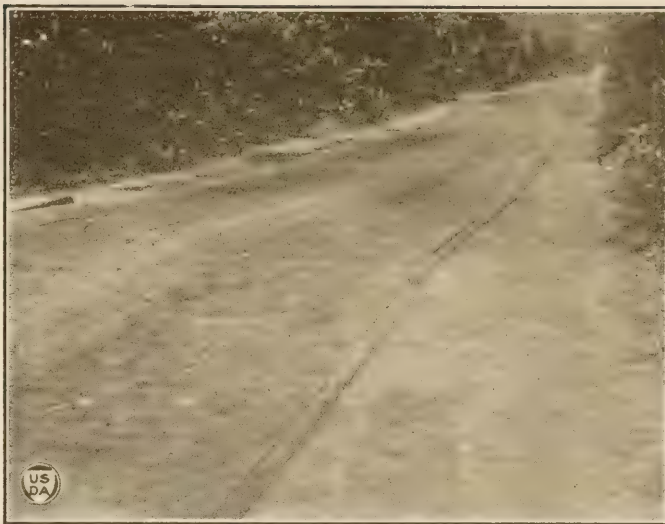
Fig. 23.—Section of a cement-grout-filled surface laid through a swamp section south of Kissimmee which has conformed to changes in the sand subgrade without becoming rough.
