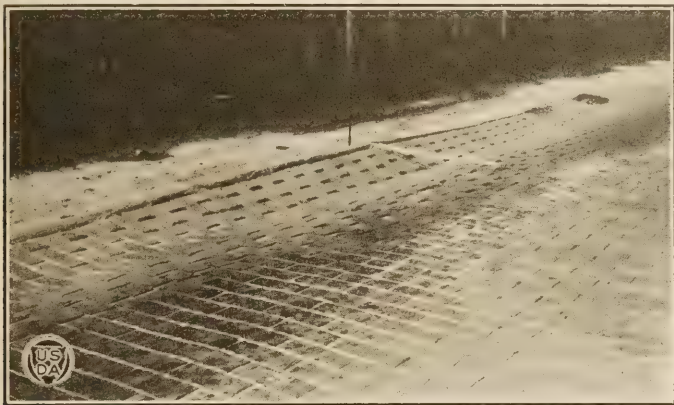
Fig. 21.—Depression in Orlando-Winter Garden road, probably caused by displacement of the sand subgrade, due to vertical movement of the curb.
