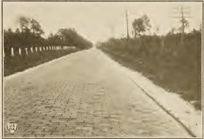
FIG. 2.—State Route No. 1 between Jacksonville and Lake City, showing lack of "beam strength."
