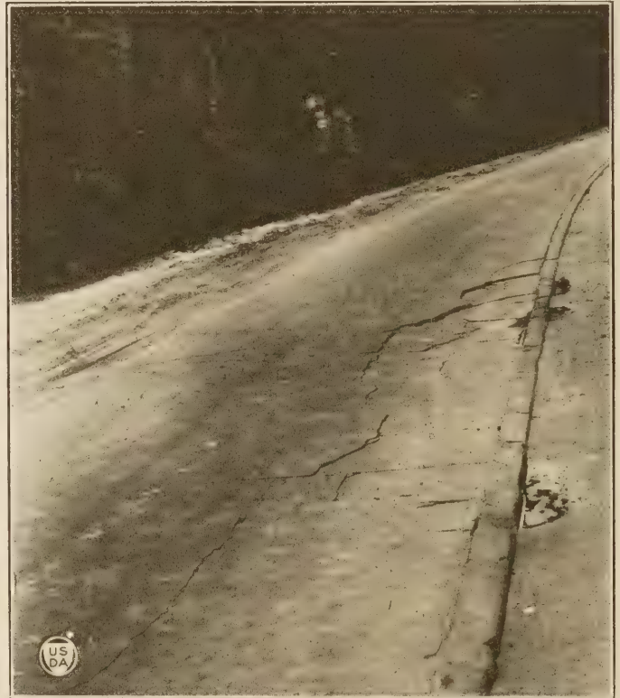
FIG. 6.—Break on curve of cement-grout-filled surface—State Route No. 2, between Orlando and Sanford.
