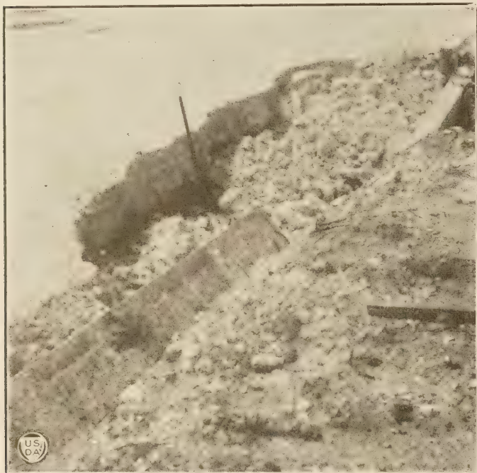
FIG. 25.—Failure of limerock base due to washout of sand subgrade. Note the smooth surface obtained by rolling.
