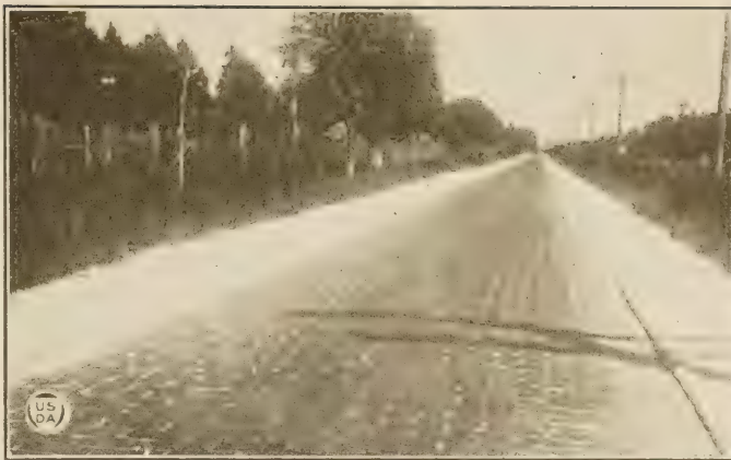
FIG. 15.—Showing settlement in a narrow, sand-filled surface laid on a shell base. This is a section of the Jacksonville-St. Augustine road.
